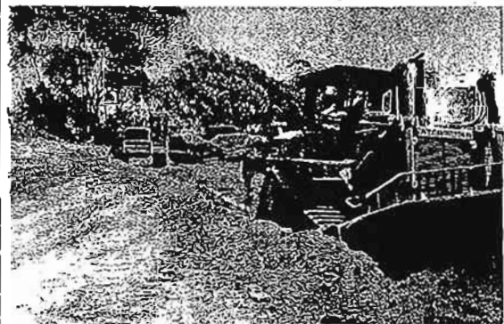
Photo 100 Grading operations in order to move the soccer field to the east.
