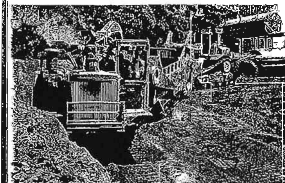
Photo 101 Grading operations near the ash pit excavation. The ash pit is located to the right of the photograph.
