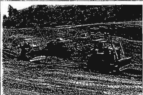
Photo 42 Large round boulders were uncovered at the tennis court over-excavation area.
