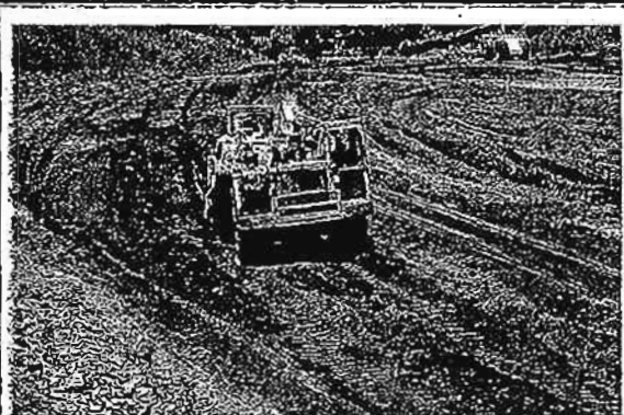
Photo 40 Over-excavation of soil where basketball courts will be constructed. The depth of cut is approx. 20 feet below ground surface.
