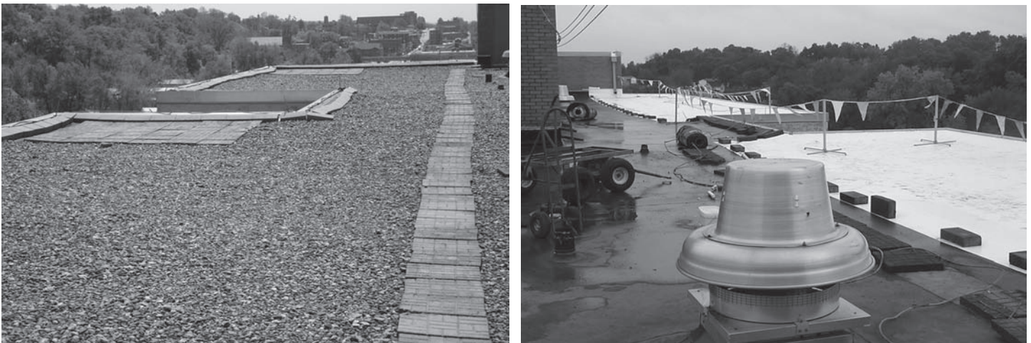
Figure 22: Roof Repairs to an Iowa Public Housing Facility, Before Work Began and Work in Progress
