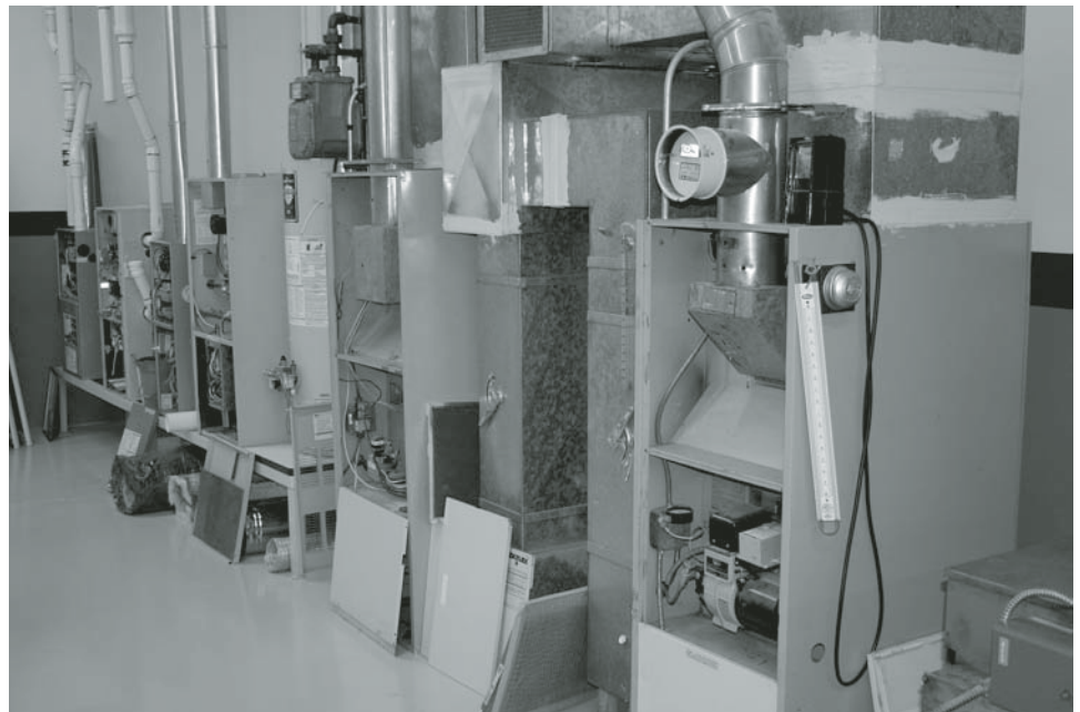
Figure 16: Heating Systems Laboratory, Weatherization Training Center at the Pennsylvania College of Technology in Williamsport, Pennsylvania
