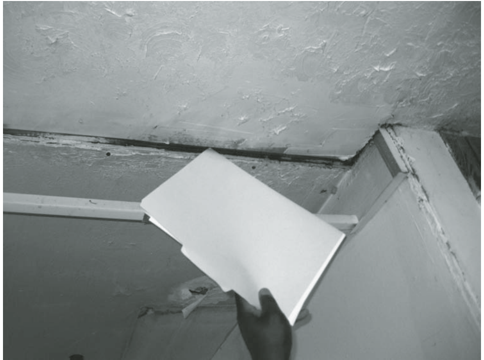
Figure 15: Pointing Out Ceiling Cracks During an Energy Audit of a Home in Georgia
