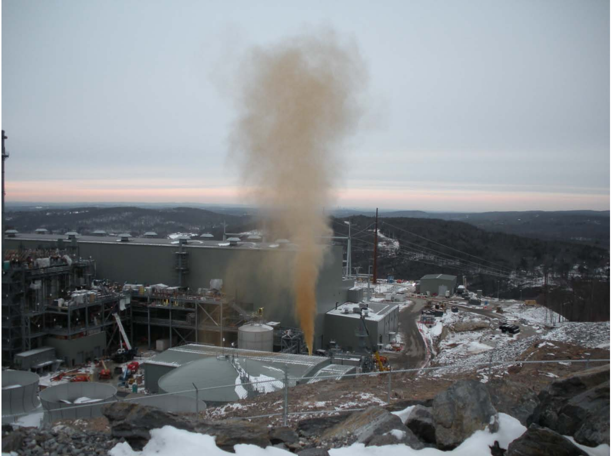
Figure 3. Natural gas blow conducted at the Kleen Energy plant a week prior to the explosion on February 7, 2010, showing plume of gas and debris hundreds of feet high.
