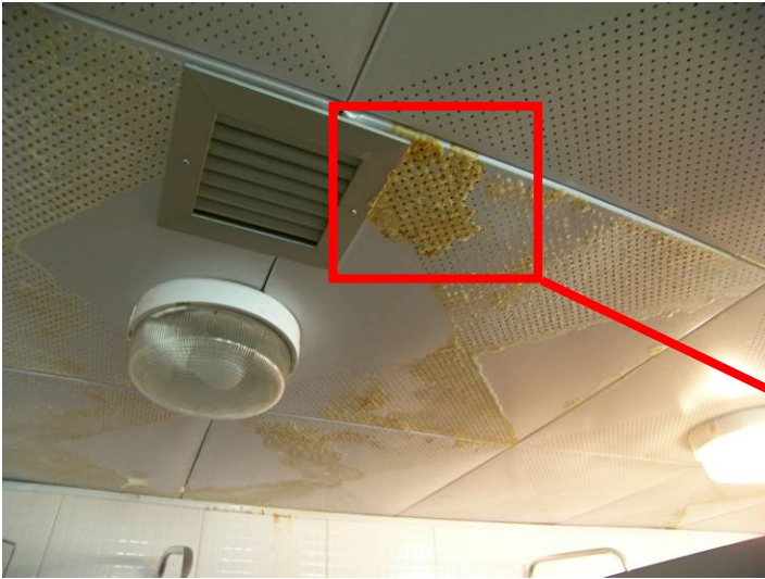
Site Photo 18. Urine stain on the second floor ceiling
