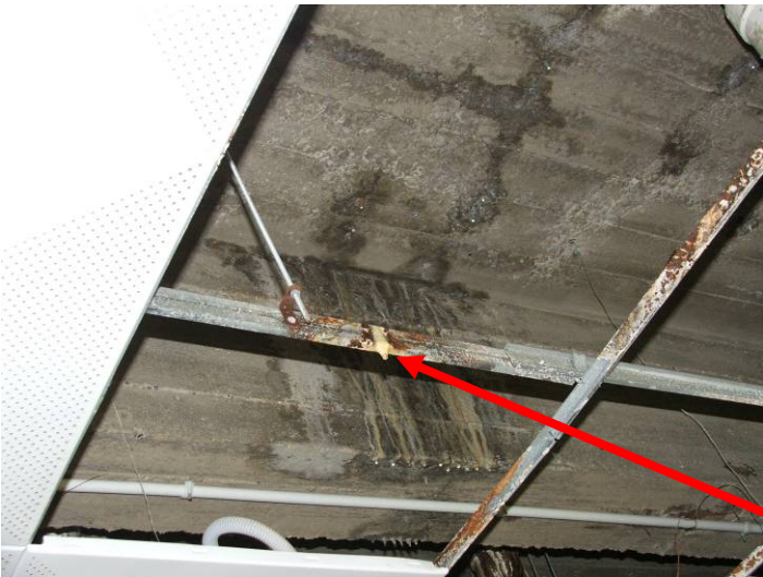
Site Photo 20. Ceiling Dripping
