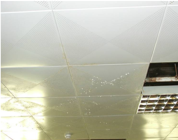
Site Photo 7. Water leaking from ceiling
