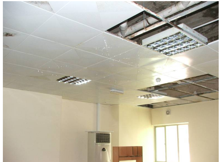
Site Photo 8. Water leaking from ceiling
