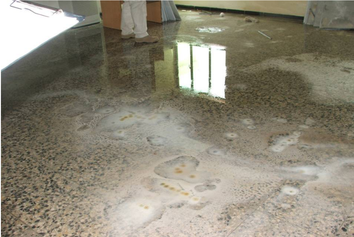
Site Photo 11. Additional view of water damage and residue from dissolved minerals and materials in the water from leaking ceiling
