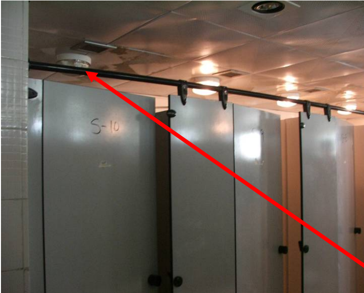
Site Photo 16. Bathroom lights on second floor
