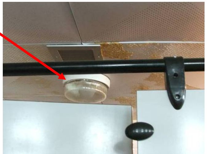
Site Photo 17. Close-up view of far left bathroom light not operating because it is full of diluted urine and fecal matter
