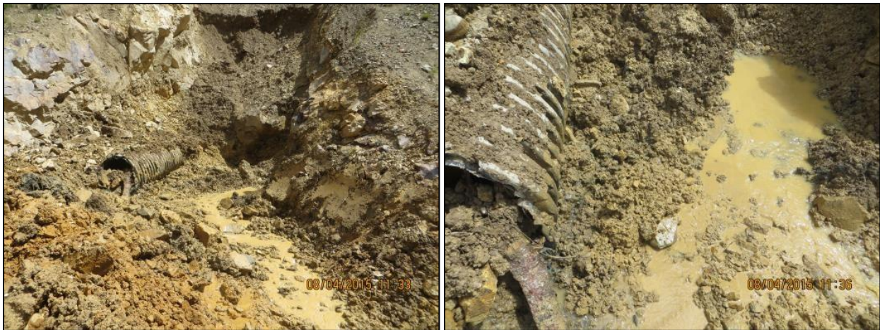
Photographs Showing Upper 24" Corrugated HDPE Observation Pipe
