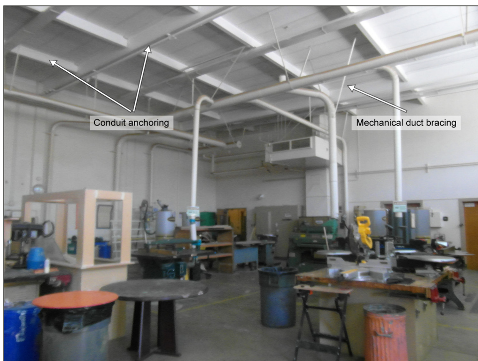
Figure 4: Anchoring and Bracing of Building Components in a Los Angeles Unified School District School Building
