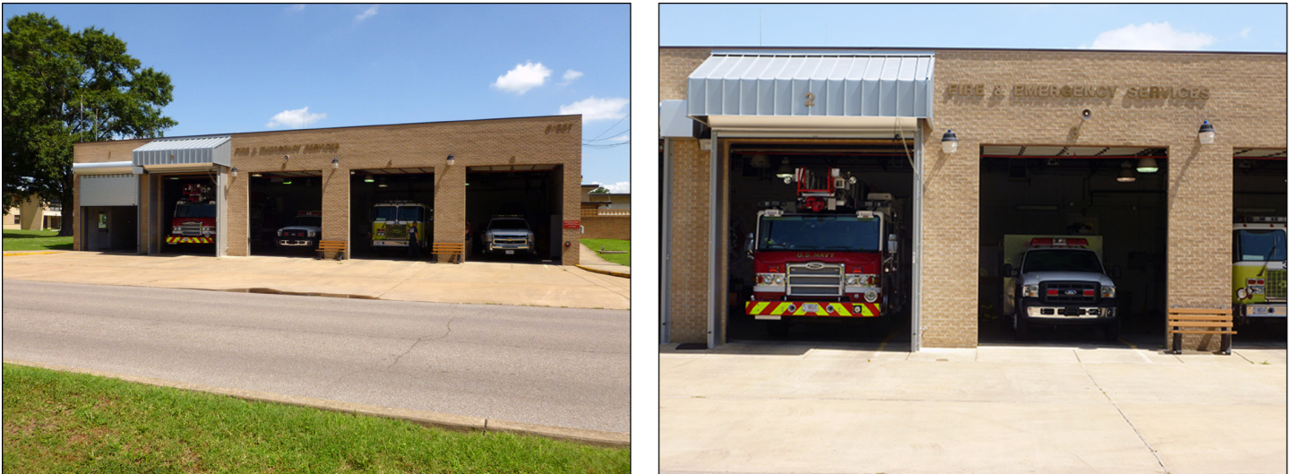
Figure 7: High Seismic Risk Unreinforced Masonry at Security and Fire Department Building on Navy Installation
