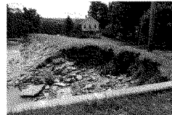
Flood damaged levee, Bainbridge, NY— Courtesy of NYSDEC
