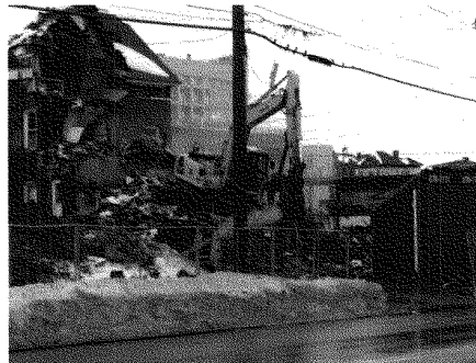
Construction of a new mixed-use development, Butternut Commons, is underway just a few blocks from where a sewer collapse has shut down Butternut Street for two weeks.
