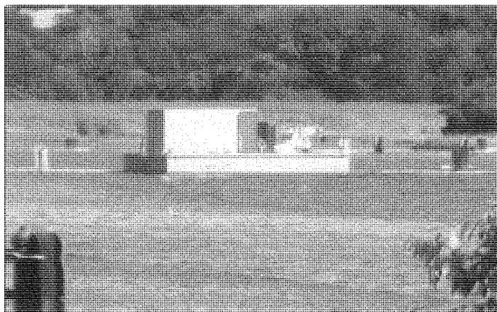
In New Bedford Harbor, Massachusetts the dredge is towed by cables from the shore
