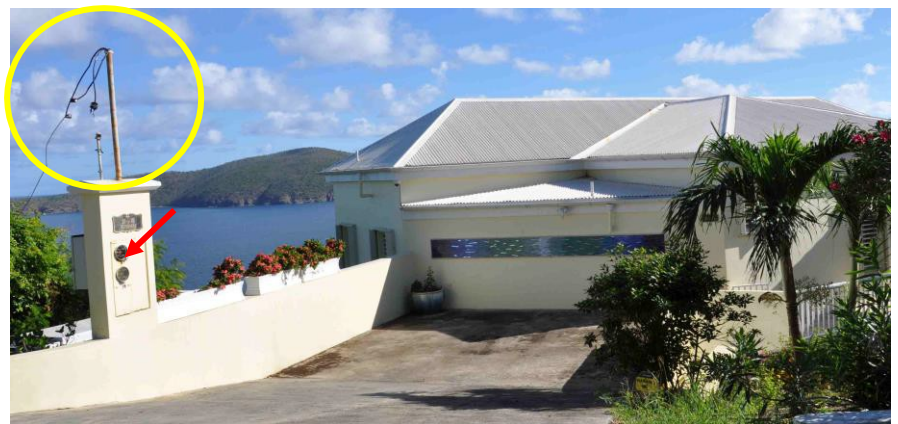
Figure 15. Overhead power line terminated at a service mast (yellow circle) anchored to a concrete pylon (red arrow). Service ran underground from the pylon to the house.
