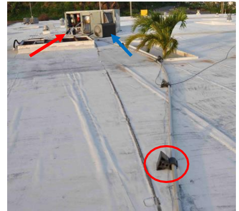
Figure 13. The displaced electrical conduit used supports (red circle) that rested on the roof. Displaced HVAC unit (red arrow) and condenser (blue arrow).
