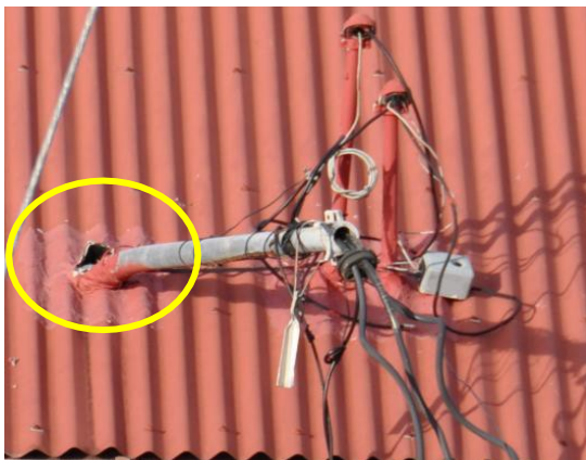
Figure 14. A collapsed overhead power line pulled over this service mast which caused flashing rupture (yellow oval).
