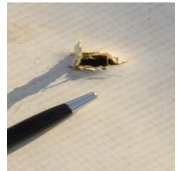
Figure 6. Punctured roof membrane at a school (pen for scale).
