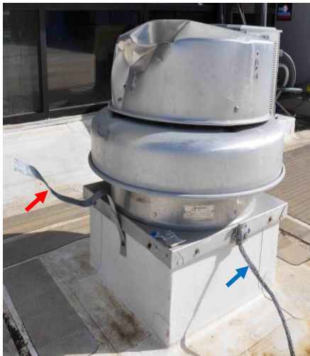
Figure 7. Damaged fan cowling with damaged strap (red arrow). Note the lightning protection system conductor (blue arrow).
