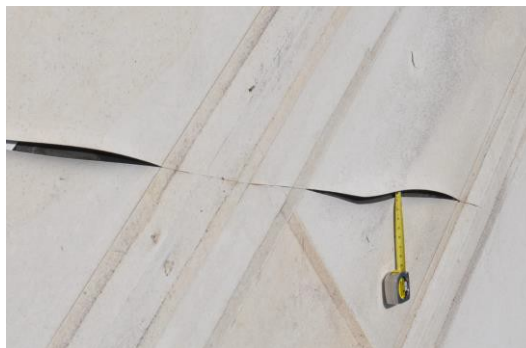
Figure 5. Torn roof membrane near the HVAC unit show in in Figure 4.
