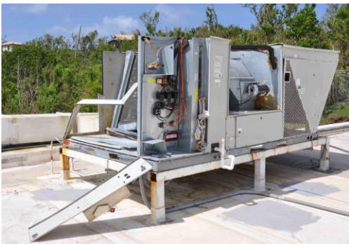
Figure 4. Blown-off unit enclosures at a medical clinic.
