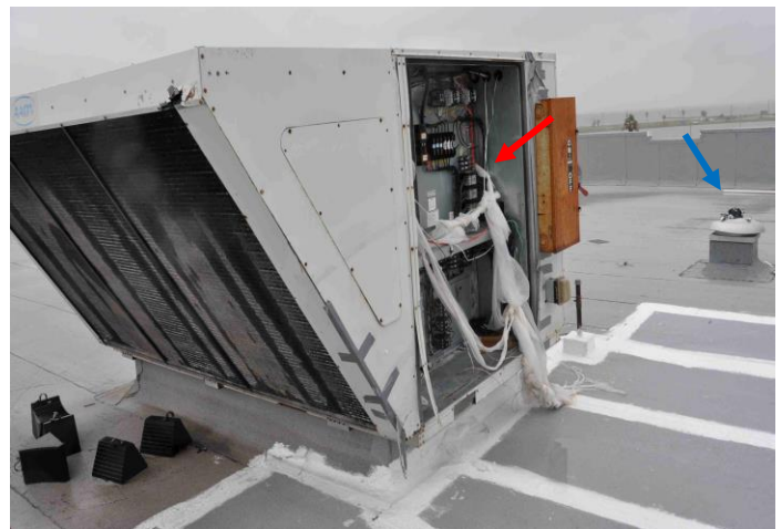
Figure 3. Blown-off access panel at a hotel (red arrow) and blown-off fan cowling (blue arrow). Hurricane Harvey, Texas.
