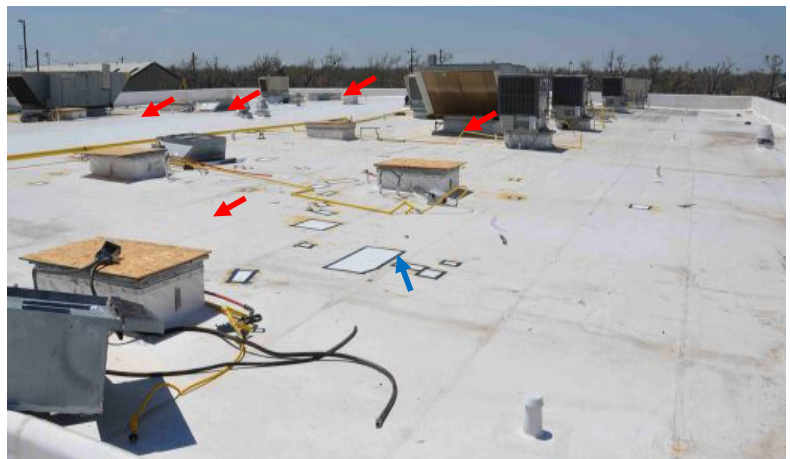
Figure 1. HVAC units blown off their curbs (red arrows). Curb openings were temporarily covered with plywood. Patches had been installed at membrane punctures (blue arrow). Hurricane Harvey, Texas.
