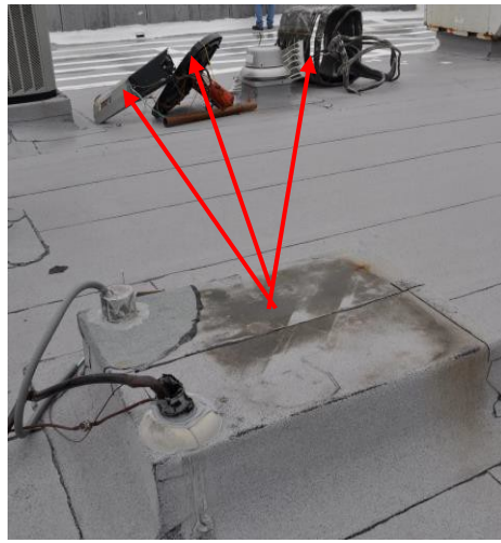
Figure 8. The condenser at this hotel was placed on the curb and was not anchored. Hurricane Harvey, Texas.
