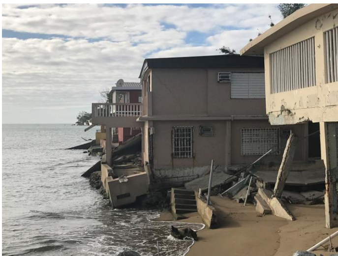
Figure 9. Structures located close to shore and subject to scour and erosion.
