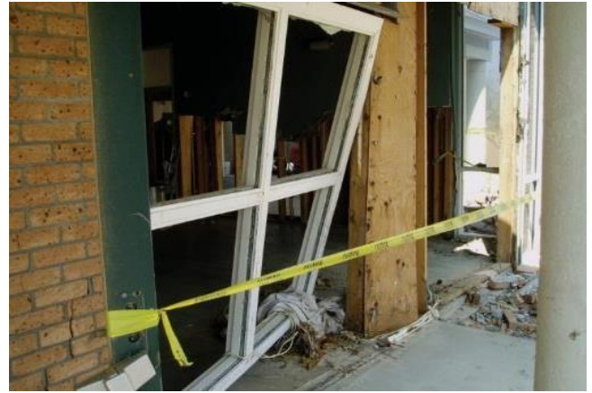
Figure 3. Failure of wood-frame wall, brick veneer, and windows due to 4 feet of stillwater flooding and small waves. Hurricane Katrina in Mississippi.
