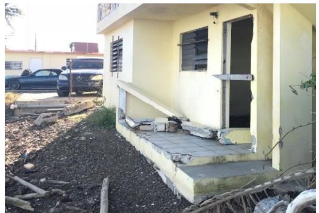
Figure 4. Failure of A Zone type foundation in a coastal area, not subject to Zone V conditions.
