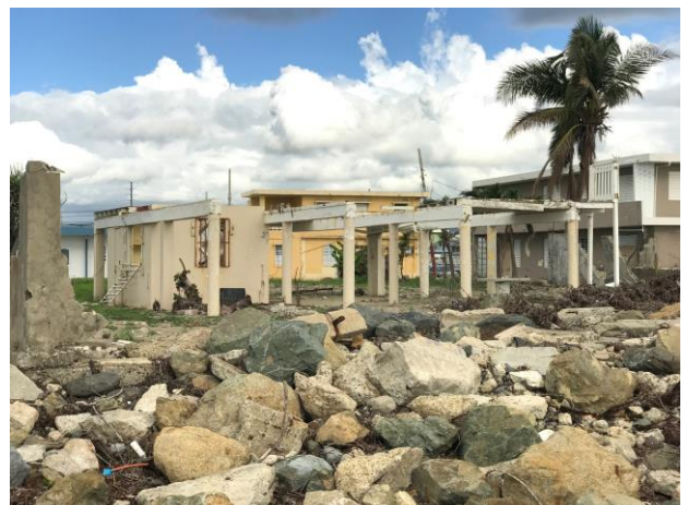
Figure 2. Severely damaged structure in Coastal Zone in Punta Santiago.
