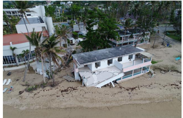
Figure 1. Failure of structure subject to surge, waves, and erosion.
