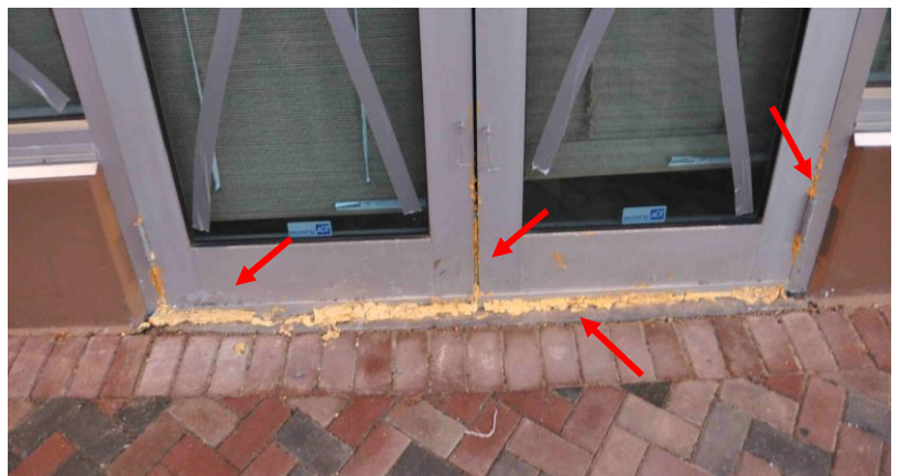
Figure 1. Expanding foam insulation was applied at gaps around and between these doors (red arrows).
