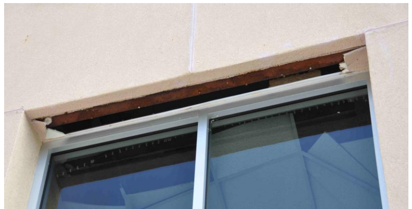
Figure 6. Blow-off of the wall covering at the window head recess at a hospital allowed entrance of wind-driven rain.
