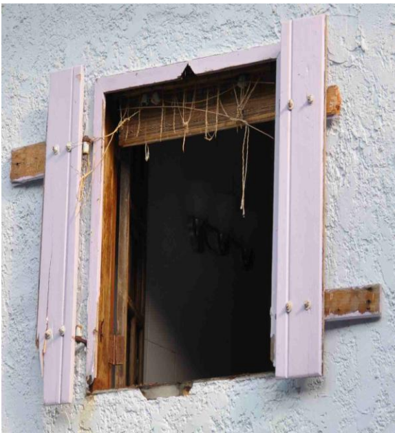
Figure 9. Damaged traditional-type shutter.
