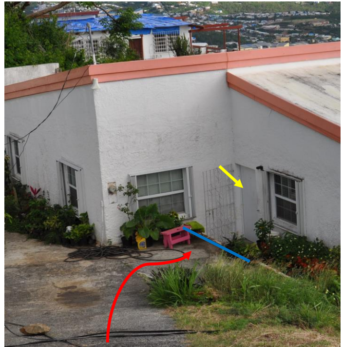
Figure 3. A substantial amount of water entered this house at the door (yellow arrow). The curb (blue line) was too short to divert the water running down the driveway.
