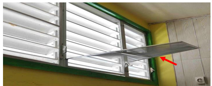
Figure 5. Glazed panels (red arrow) were mounted to the inside the jalousie. Such panels are typically ineffective in preventing entry of wind-driven rain.
