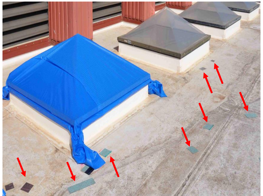
Figure 10. Skylight damaged by wind-borne debris. The red arrows indicate patches where debris punctured the roof membrane.
