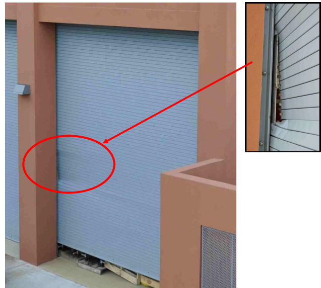
Figure 2. Rolling door damage at a new fire station.
