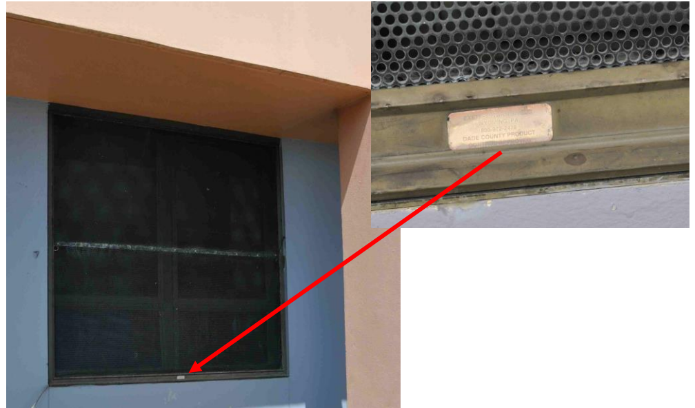
Figure 8. Permanently mounted wind-borne debris-resistant screen at a medical clinic. The inset shows a close-up of the screen and a label indicating that the shutter was a tested assembly.
