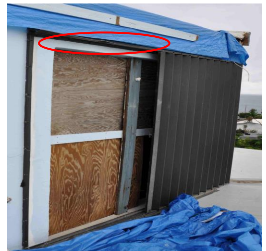
Figure 7. The red oval indicates where the head track was deformed. Plywood was temporarily installed after the storm.
