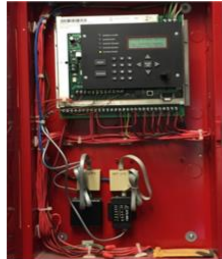
Automatic Sprinkler System Panel
