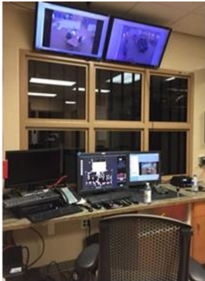
Oglala Sioux Tribal Offenders Detention Center Control Room, Pine Ridge, SD
