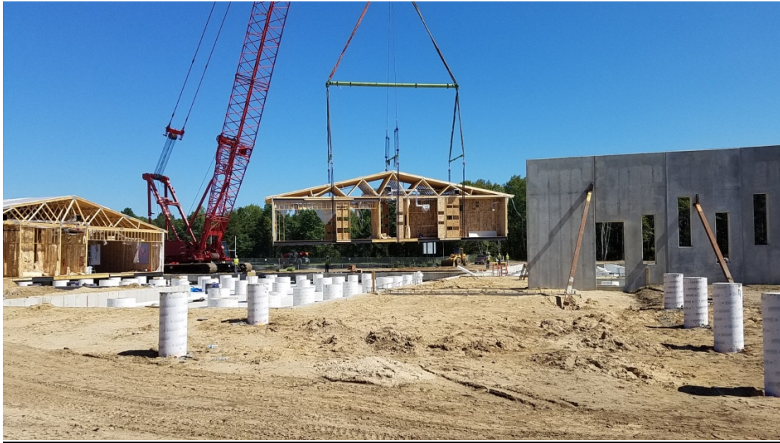
Placing a Module On-Site for the Construction of the Bug-O-Nay-Ge-Shig High School in MN
