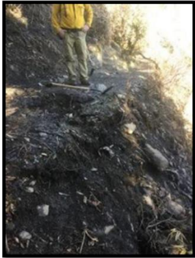
Public trails became unstable where the wildfire burned on hillsides, posing grave danger for hikers.
