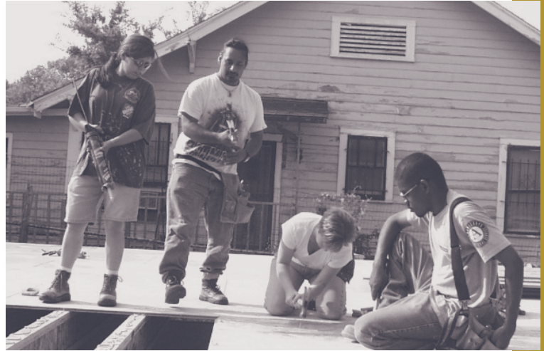
American YouthWorks AmeriCorps (Casa Verde Builders) volunteers building the floor of a new house. (Photo courtesy of American Youth Works)
