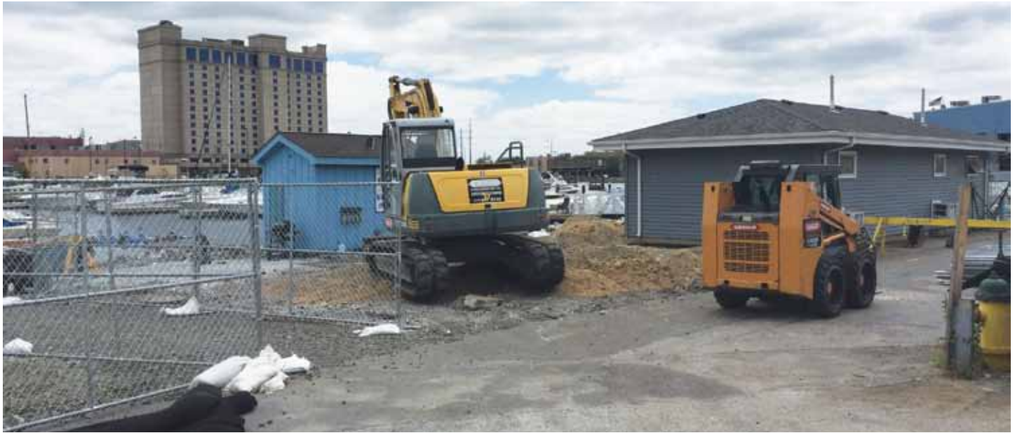
Work underway at the marina in East Chicago in the summer of 2017.
