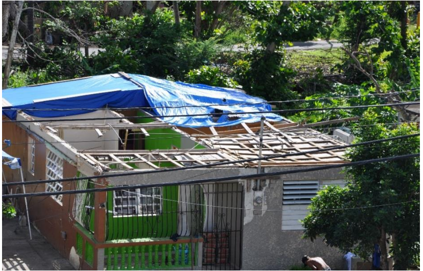
Figure 2. A damaged corrugated metal roof. The roof did not have plywood sheathing or adequate roof support framing or connections.
