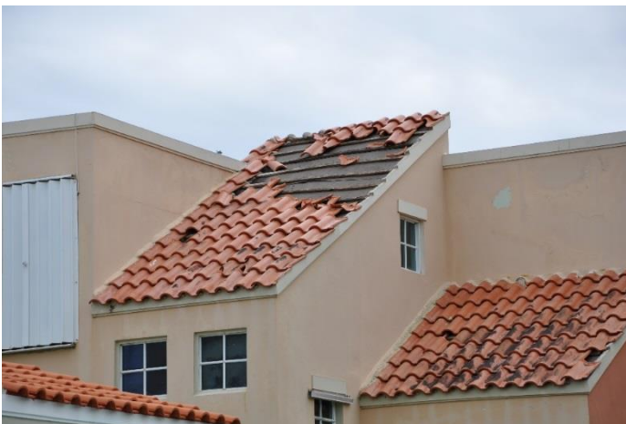
Figure 3. A damaged clay tile roof.
