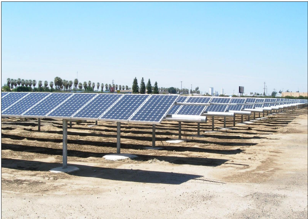
Figure 7: Example of a Ground-Mounted Solar PV Installation
