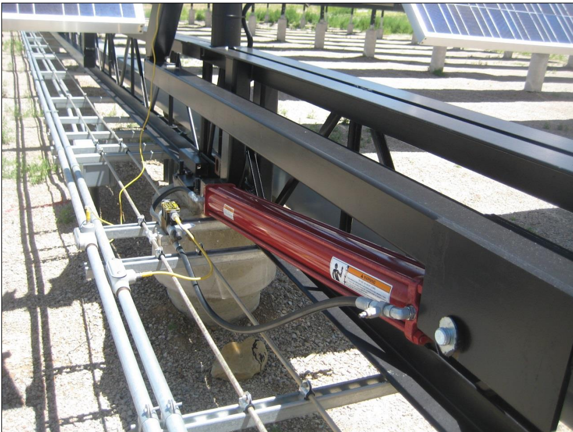
Figure 8: Example of a Tracking Solar PV Installation
