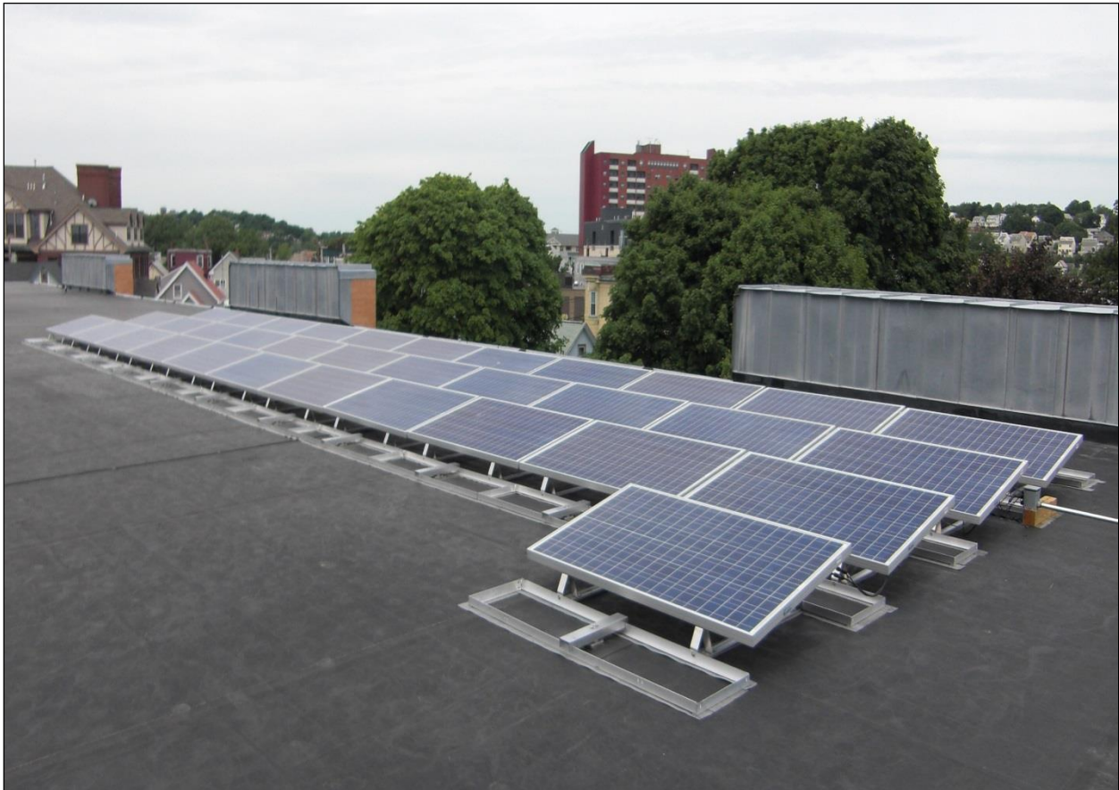
Figure 6: Example of a Roof-Mounted Solar PV System
