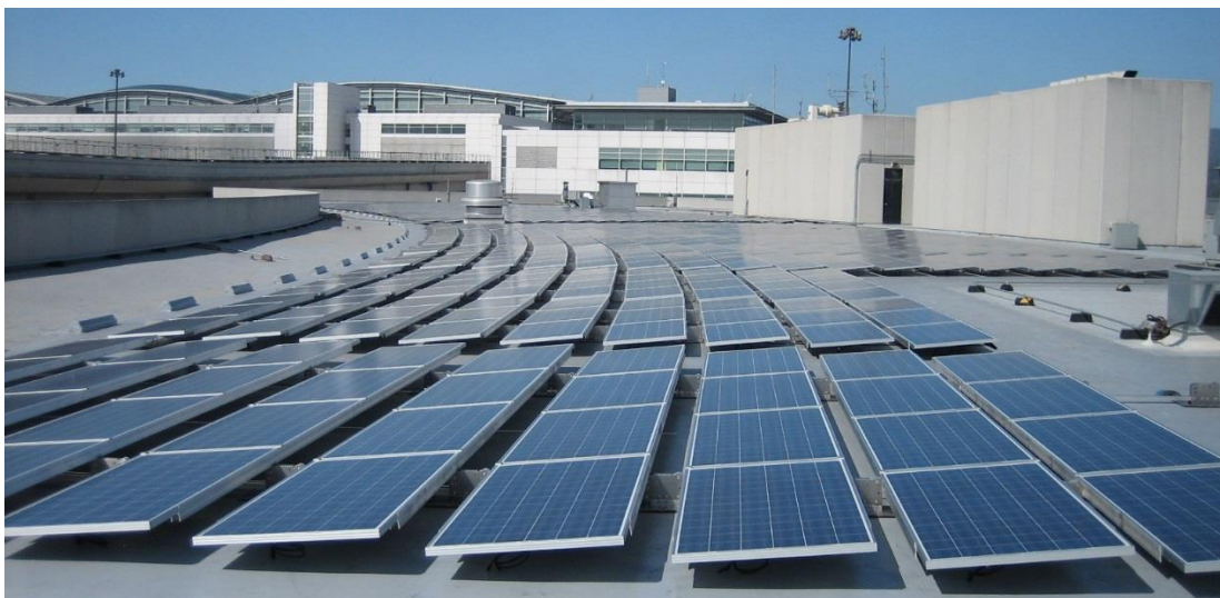
Figure 24: Rooftop Solar Project on San Francisco’s Terminal 3
