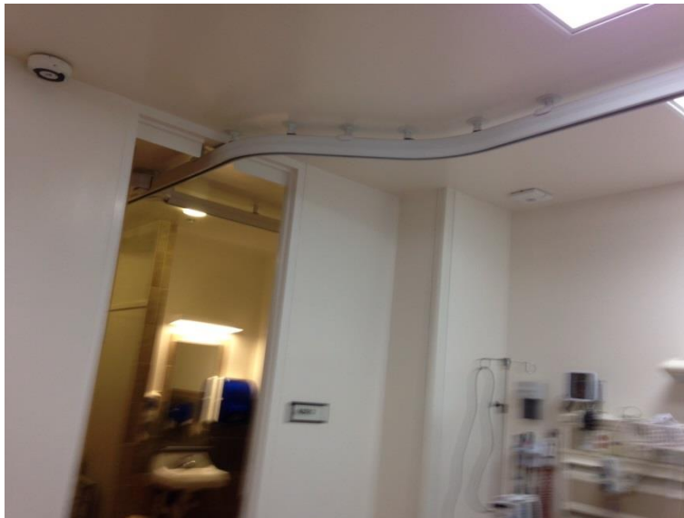
Figure 5. Overhead lift track connecting into bathroom with a turntable in the bathroom
