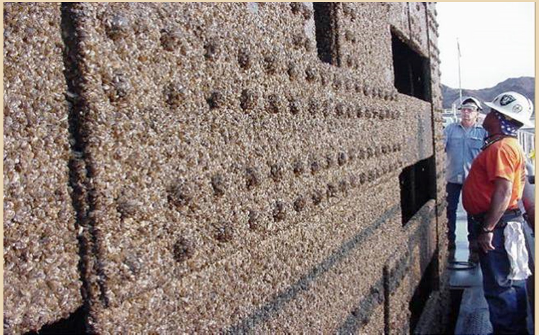
Bulkhead Gate inspection of invasive mussels at Davis Dam, Lower Colorado Region in October 2007. Invasive mussels were found in Lake Mead, also of the Lower Colorado Region, in January 2007. This gate at Davis is 67 miles downstream from Lake Mead.
