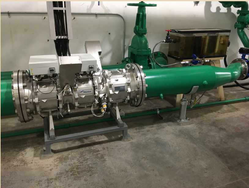
UV unit installed at Parker Dam (Lower Colorado River, California-Arizona).
