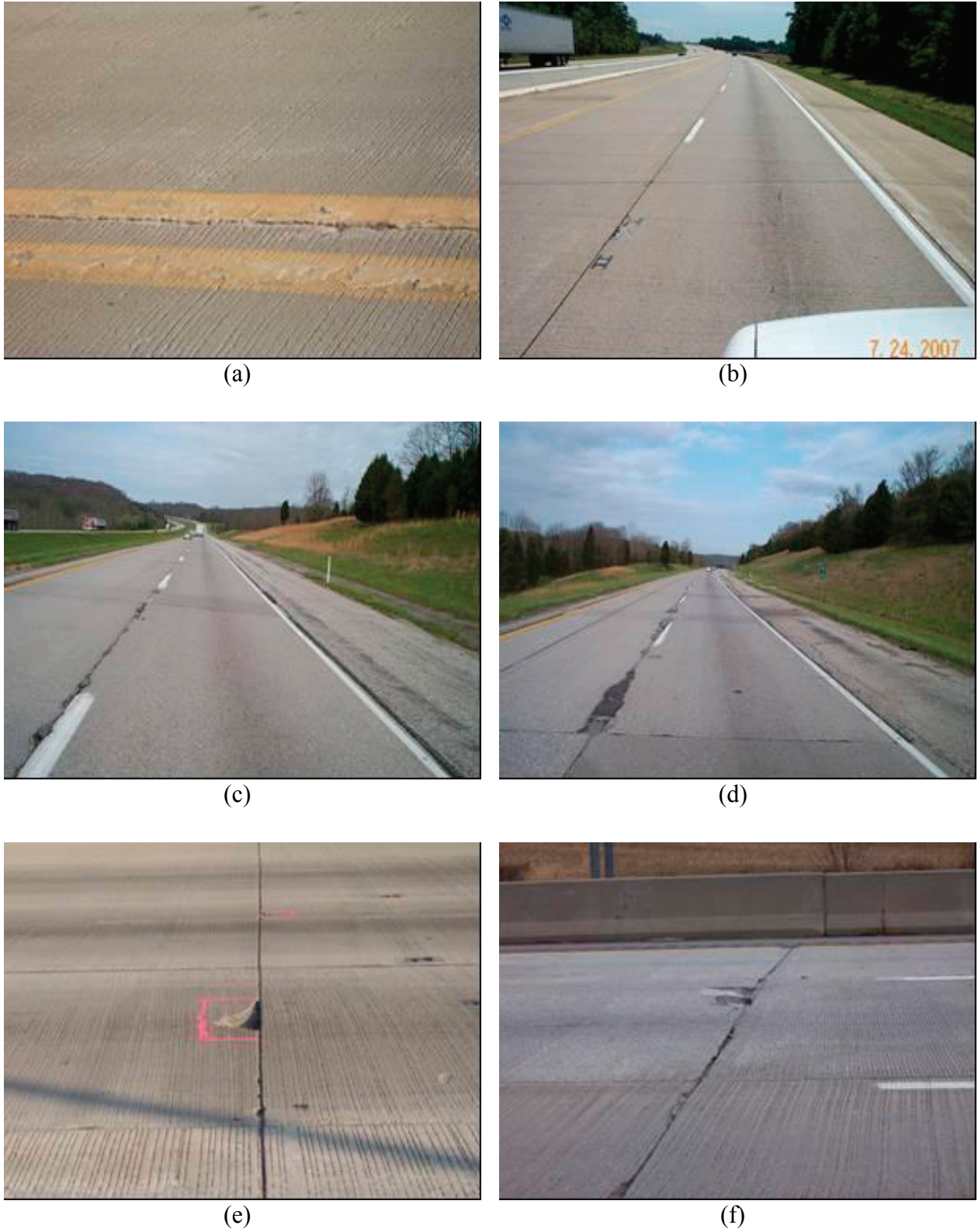
FIGURE 3-18 Spalling of joints: (a) and (b) low severity; (c) moderate severity; (d), (e), and (f) high severity
