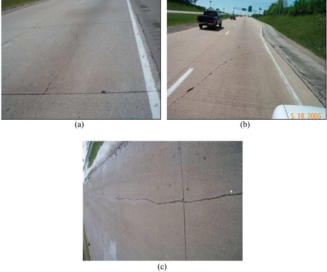
FIGURE 3-17 Longitudinal cracking: (a) low severity; (b) moderate severity; (c) high severity
