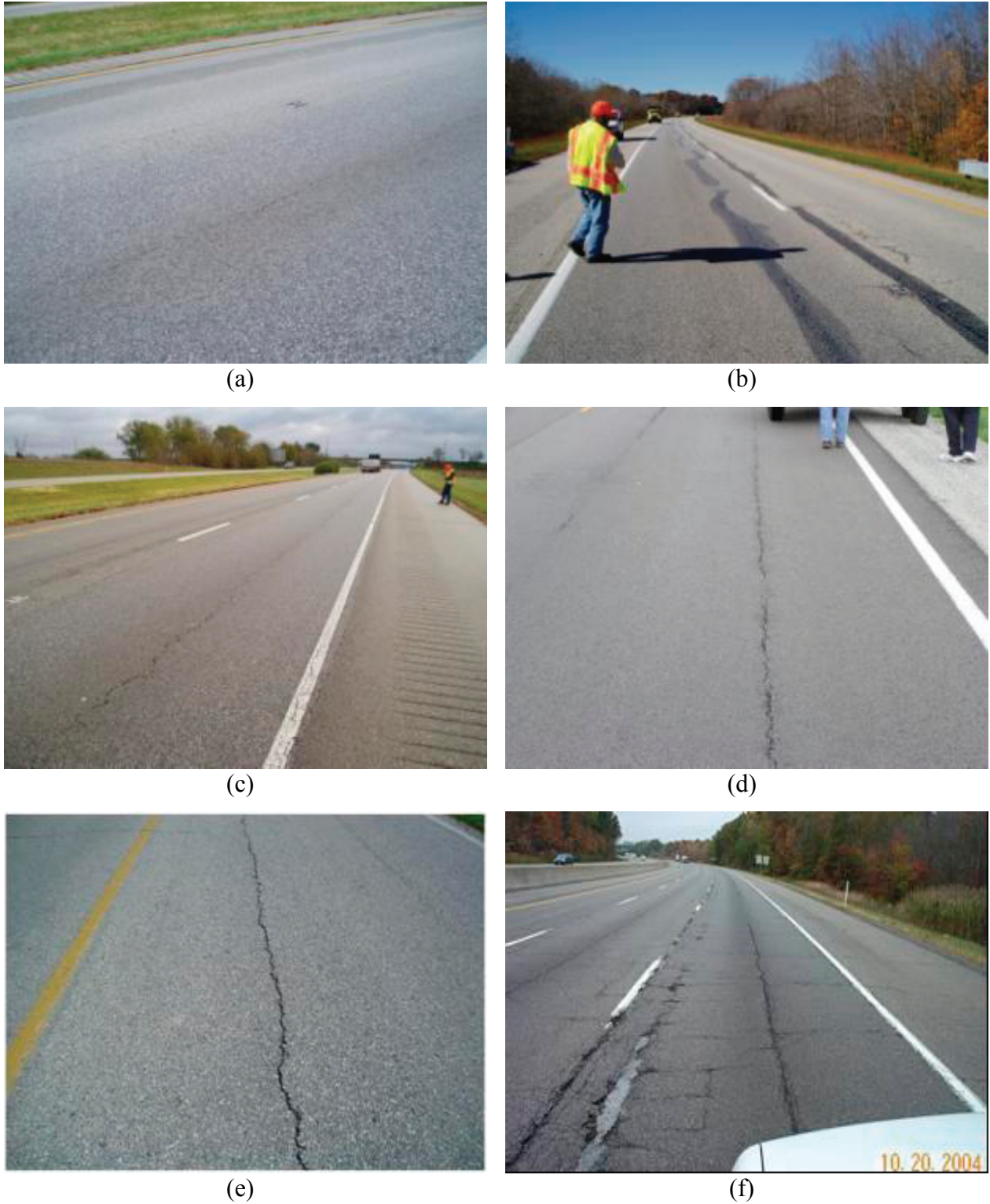
FIGURE 3-3 Longitudinal cracking: (a), (b), (c), and (d) low severity; (e) moderate severity; (f) high severity
