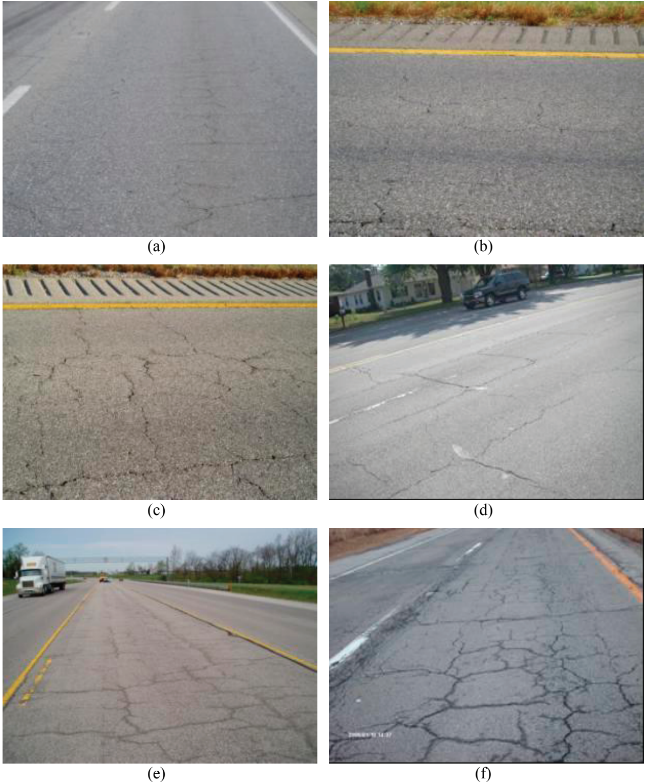
FIGURE 3-5 Block cracking: (a) low severity; (b), (c), (d), and (e) moderate severity; (f) high severity
