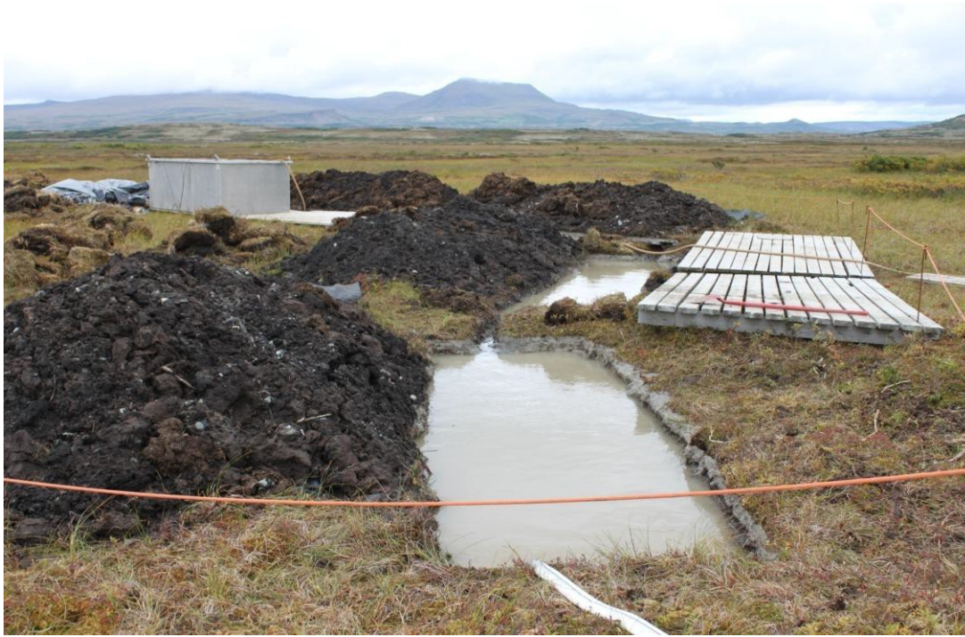
Figure 3. Excavated settling ponds (sumps) located at the PLP rig platform shown in Figures 1 and 2. Sumps are approximately 5' deep, 8' wide, and 10' long. Operation is pumping drilling muds (such as bentonite) and drilling fluids and additives into the sumps. The drilling muds and fluids are coating the walls of the holes. Photographer Rick Halford, September 1, 2011.
