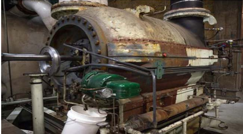
Chiller reaching the end of its life expectancy.
