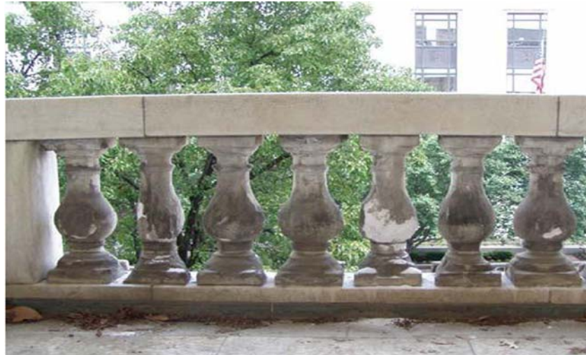
Stone sugaring on the Russell Senate Office Building balustrade.
