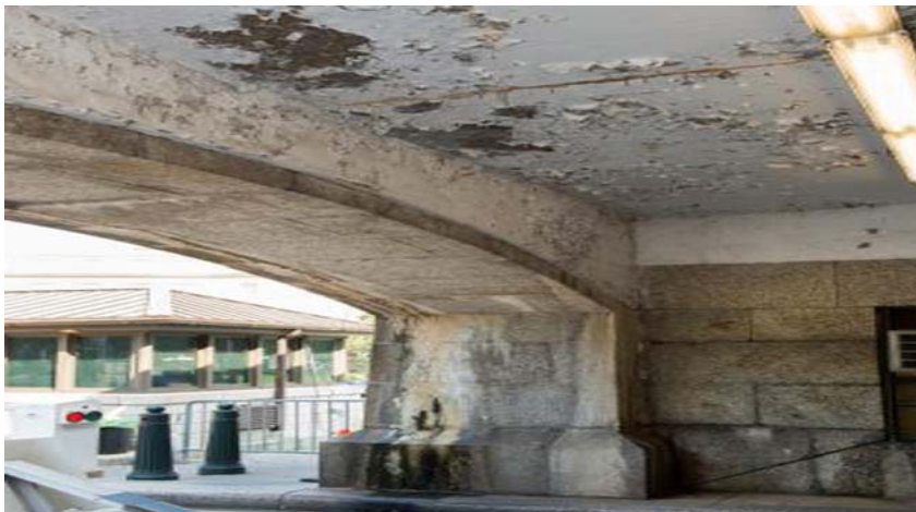
Deteriorated Senate Underground Garage.
