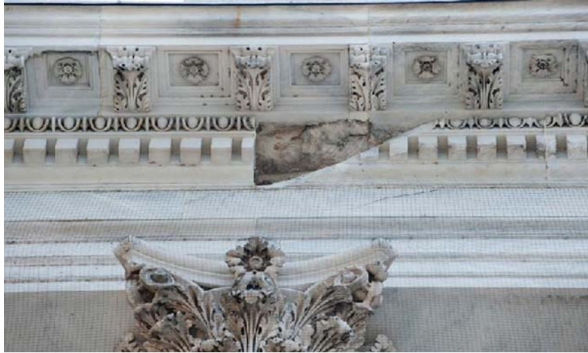
Spalling stone on the U.S. Capitol Building.
