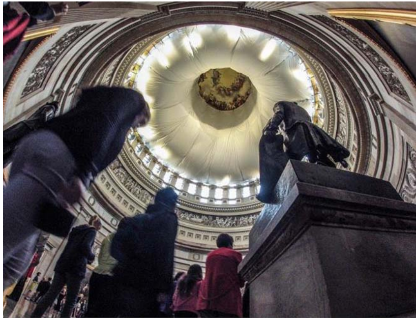
Safety canopy over the Rotunda in support of the Capitol Dome Restoration.
