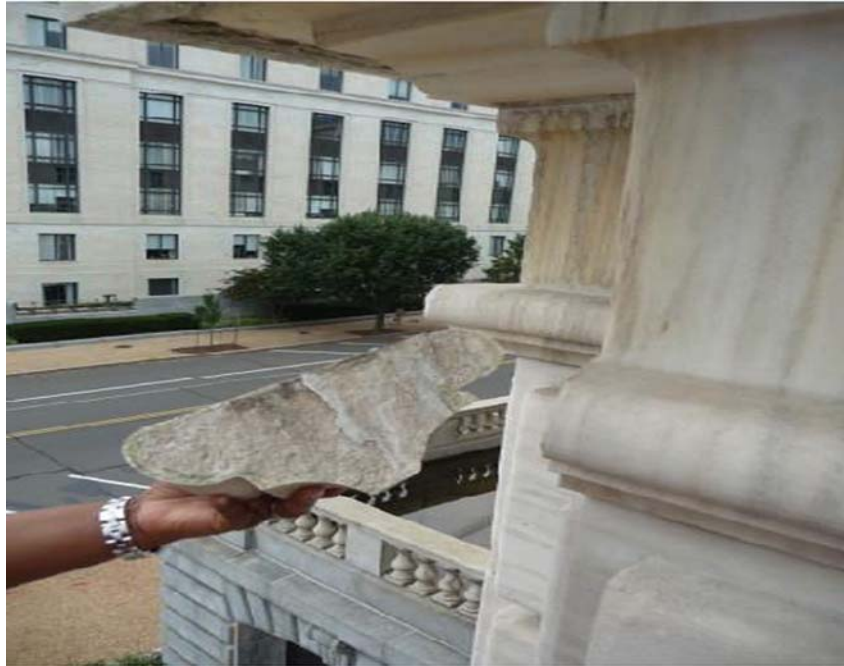
Deteriorating stone on the Russell Senate Office Building exterior.
