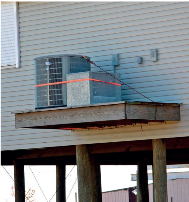
Figure 7. A cantilevered platform to elevate a residential air conditioning compressor and protect it from flooding. From FEMA P-348 (Figure 3-2).
