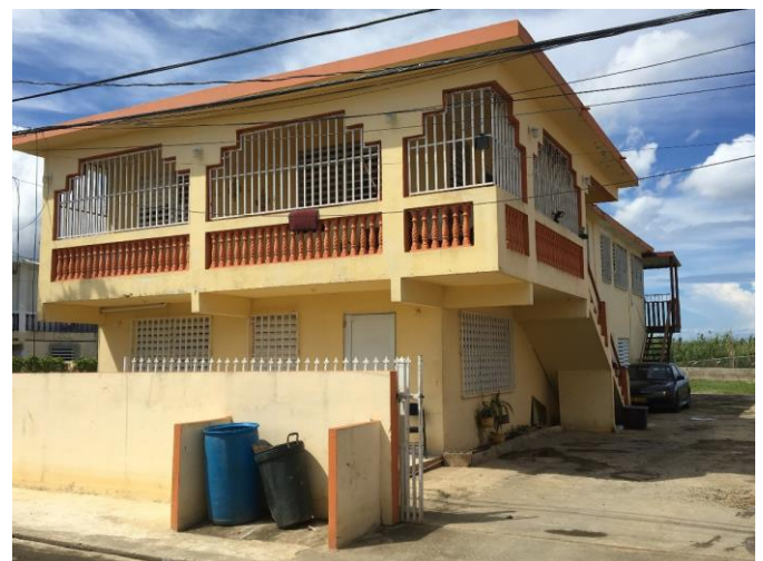
Figure 2. Typical concrete frame residential structure with a concrete roof in Vega Baja.
