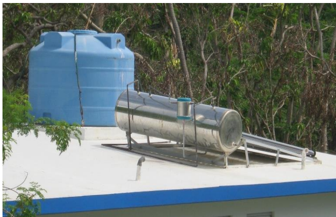
Figure 4. Solar water heater and water tank anchored to concrete roof in Rincon.
