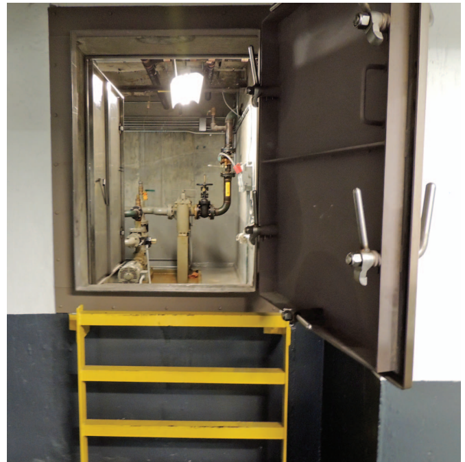
Figure 8. Example of dry floodproofed vault used to protect fuel pump equipment in a high-rise building. From FEMA P-942, RA-6 (Figure 1).
