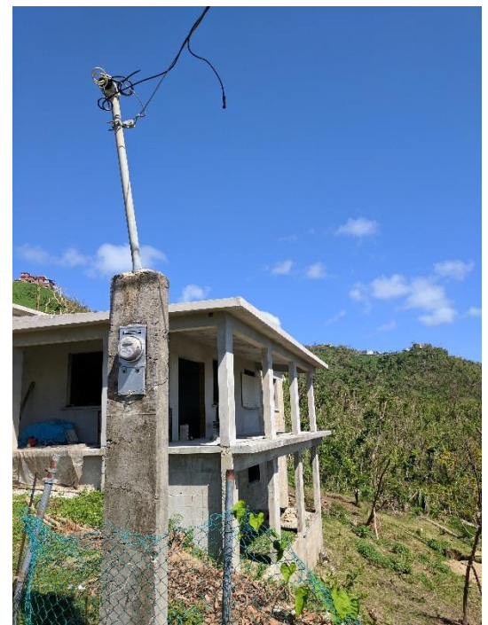
Figure 5. Electric meter elevated on concrete mast in house under construction in Yabucoa.
