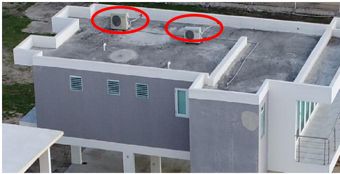
Figure 9. Heating, Ventilation, and Cooling (HVAC) equipment (red ovals) anchored to concrete roof deck in Humacao.
