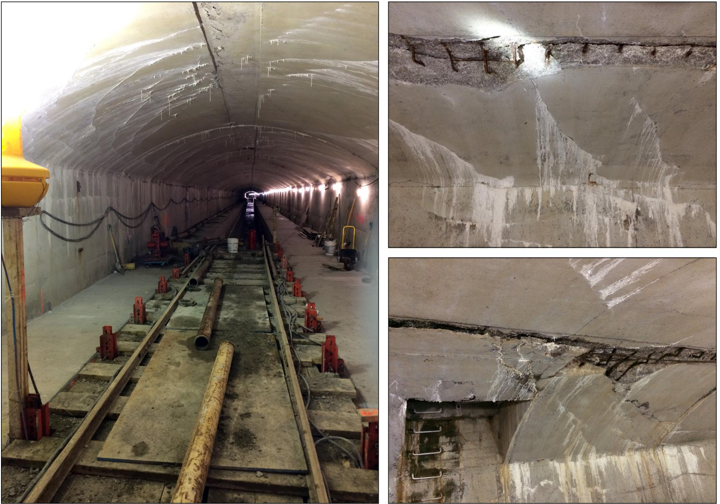
Figure 6: Damage to the Mountain Trunk Storm Sewer, City of Hamilton, Ontario, Canada
