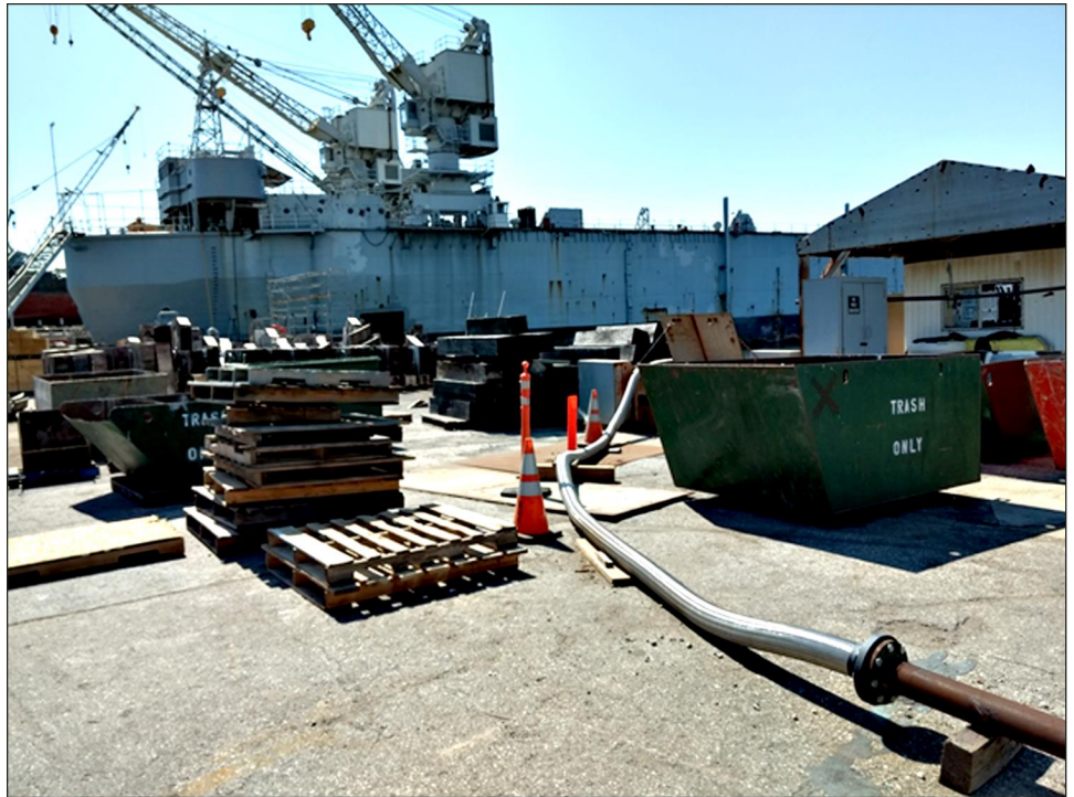
Figure 4: Temporary Steam Heating Pipe Running through Dockside Equipment, U.S. Coast Guard Yard, Curtis Bay, MD
