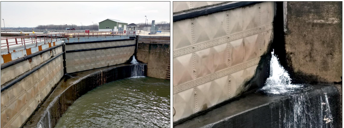
Closed lock gates with water leak in lower right-hand corner, Brandon Road Lock and Dam, Joliet, IL
