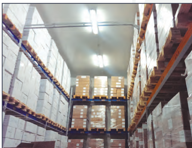
The central deposit cold room in Casablanca, Morocco.
