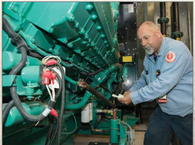
Jon Stelzner, a Facility Management electrician, checks the oil in an emergency generator in the medical center. FM staff design, build and maintain most of what you see — and many times, don't see — on campus.
