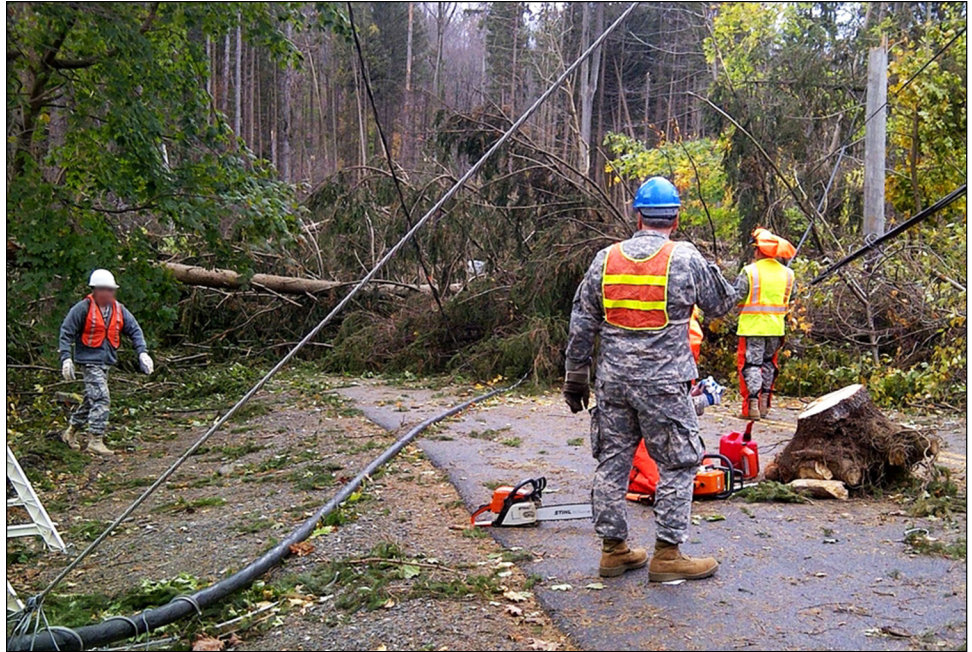
Figure 1: New York Army National Guard Engineers Clear Debris from Roads in New York State after Superstorm Sandy
