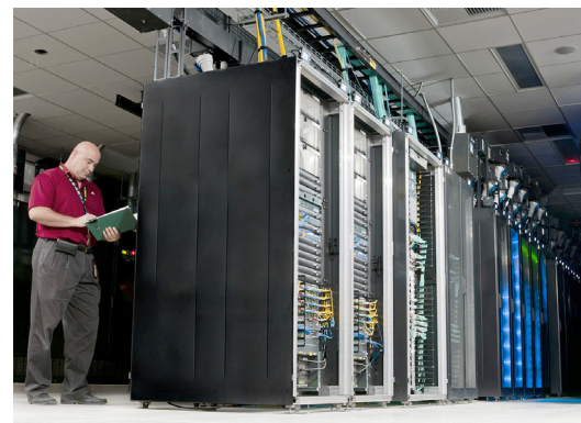
Dan Oleyar collects data center metrics at the Advanced Technology Research Facility at the Frederick National Laboratory for Cancer Research in Frederick, Maryland.
