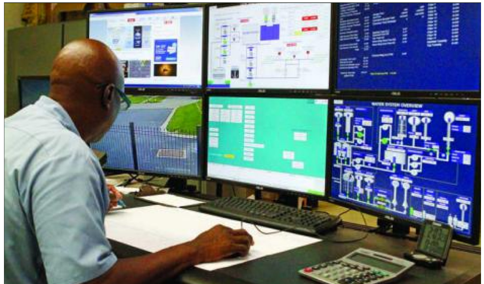
Figure 2: Wastewater Plant Treatment Operator Reviewing Supervisory Control and Data Acquisition System
