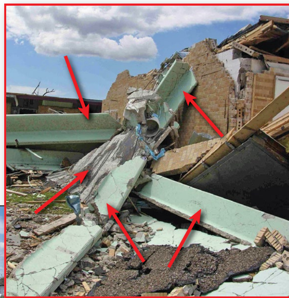
Figure B8-6. Large debris: Roof precast twin tees (red arrows) blew off a hospital and struck another portion of the building (see inset; yellow arrow shows direction of view). One of these flew approximately 80 feet. The building damage at this site was indicative of an EF3 tornado.
