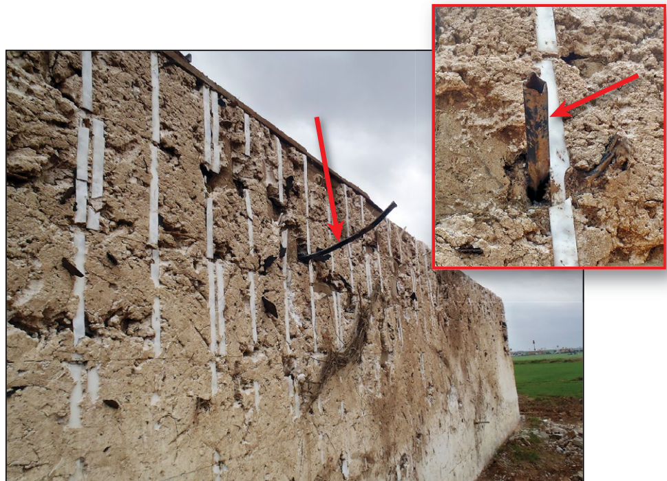
Figure B8 22. Red arrows show a steel tube that perforated a waffle grid ICF wall. Inset shows the tube in the “as found” condition and main photograph shows the tube after it was partially pulled out of the wall. (Moore, OK, 2013 tornado) (SOURCE: FEMA P-1020)
