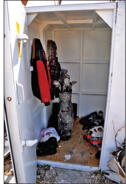
Figure B1-4. Safe room with items stored inside; such items take up space and reduce occupant capacity (Joplin, MO)
