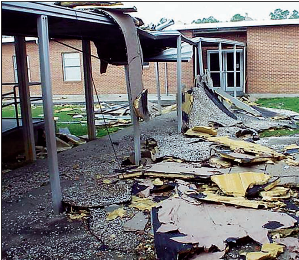
Figure B8-2. Medium debris: Pieces of a built-up roof from Hurricane Katrina (MS, 2005)
