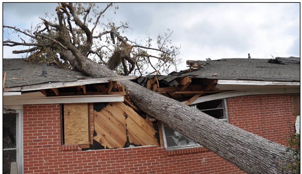
Figure B8-9. Large debris: Laydown of a large tree onto a nursing home. (Tuscaloosa, AL, 2011 tornado) (SOURCE: FEMA P-908, RECOVERY ADVISORY 6)
