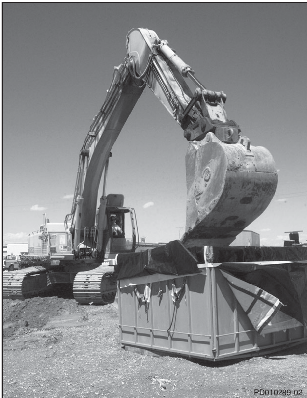
Contaminated soil is removed from a site at the Central Facilities Area.
