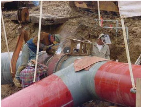
Williams-Transco engineers weld new 36" internal inspection device receiver to natural gas pipeline.
