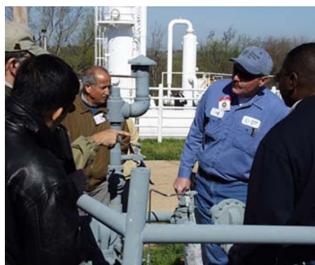
Hossein Monfared, OPS Western Region, and Jeff Harris, Oklahoma Natural Gas employee, performing a simulated inspection during a TSI field trip at a working regulator station.
