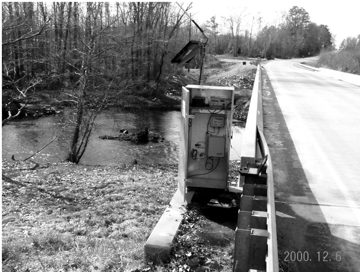
Gaging station at Swift Creek at Hilliardston, North Carolina.
