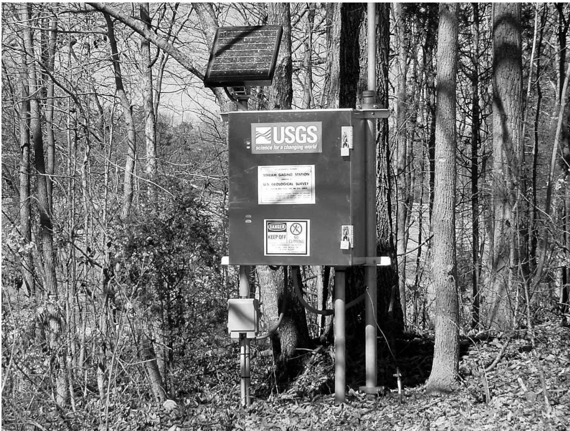
Gaging station at Long Creek near Rhyne, North Carolina.
