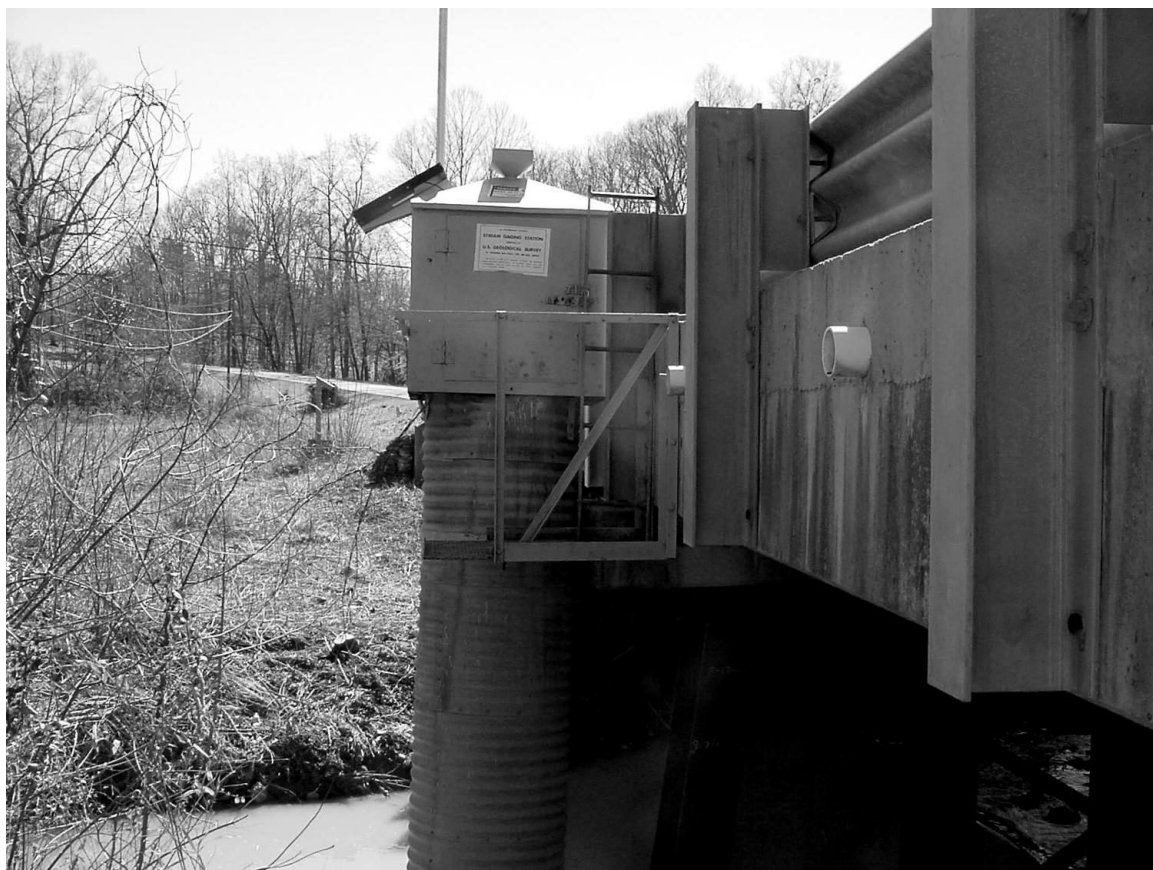
Gaging station at Long Creek near Paw Creek, North Carolina.
