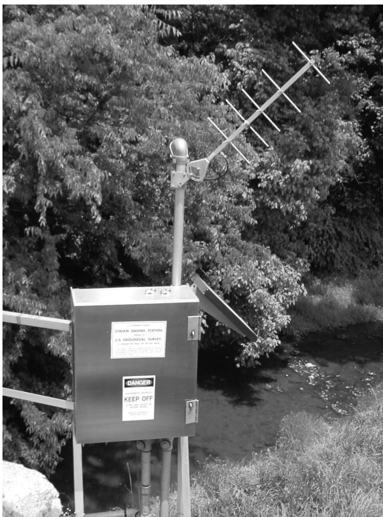
Gaging station at Goose Creek at Fairview, North Carolina.
