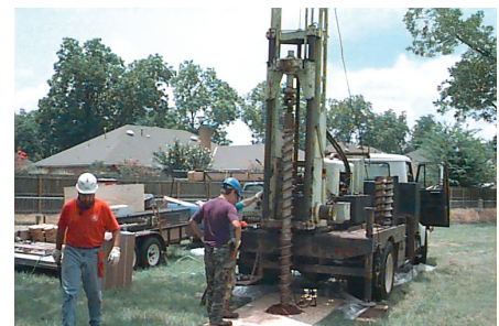
Shallow monitoring wells were installed for the urban and agricultural studies in the Mobile River Basin.
