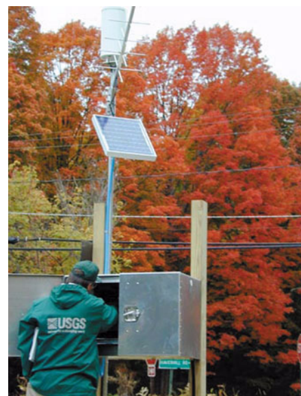
Photograph shows a hydrologist checking the equipment in a new stream-gaging station in New Hampshire.
