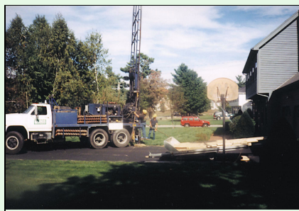
USGS installing a shallow monitoring well in a suburban area of Nashua, N.H.
