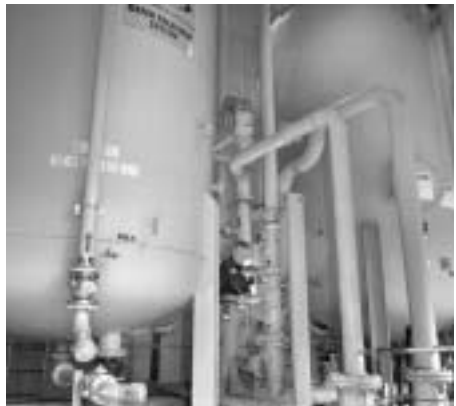
1B. CARBON FILTRATION AT WELLS 10, 11, and 12 is designed to remove volatile organic compounds before the low-iron water from these three wells directly enters the drinking-water distribution system. Noting the pressure of the carbon filtration system is Richard Lutz.
