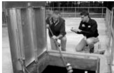
10. CLEAR WELL stores up to 250,000 gallons of what is now called "finished" water before its final chlorination and distribution. Seen taking a water sample at the clear well are Richard Lutz (left) and Jack Kulesa.
