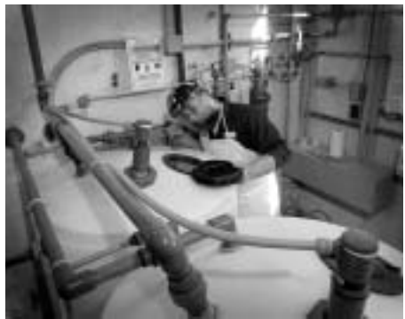
2. CHLORINATION of water from wells 4, 6, and 7 is performed at this point using sodium hypochlorite to kill bacteria and oxidize the iron in the water. Iron removal by oxidation and filtration reduces the water's iron concentration from 3 to 4 milligrams per liter (mg/l) to the "finished" water's 0.03 mg/l. Inspecting a liquid sodium hypochlorite storage tank is Joe Tullo.
