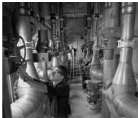
7. FILTRATION is performed, using what is called a rapid sand filter made up of eight filter cells containing sand and anthracite. Inspecting the valves in the filtration valve gallery are: (front to back) Jack Kulesa, Richard Lutz, and Steve Barcelo.
