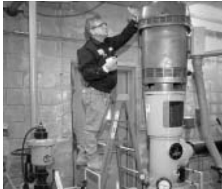
1A. WELLS 4, 6, and 7 provide source water high in iron that must be "finished" at BNL's Water Treatment Facility (WTF). At one of these wells, Phil Pizzo performs preventive maintenance on pump motor.
