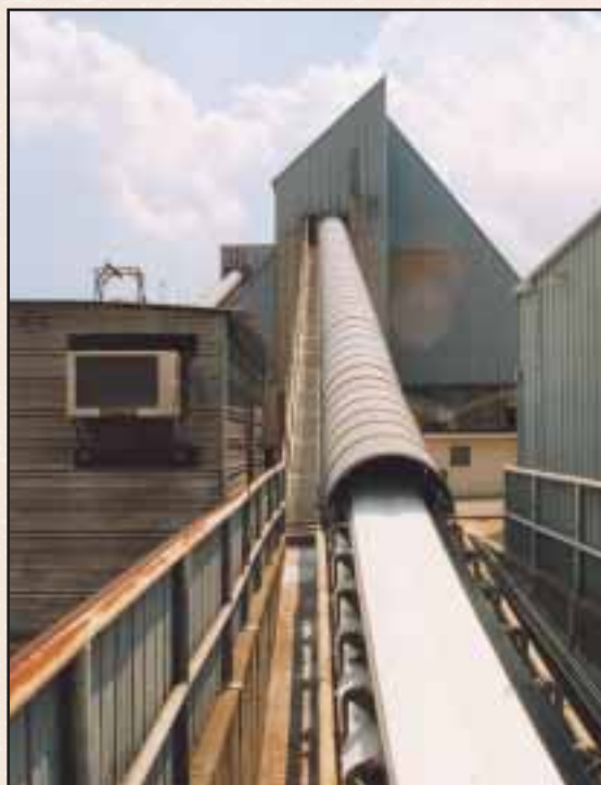
Bucket cranes unload bulk materials from ships and drop them on this conveyor belt, which terminates in a warehouse. More conveyor belts carry them from the warehouse to rail cars. Photo courtesy Port of Galveston
