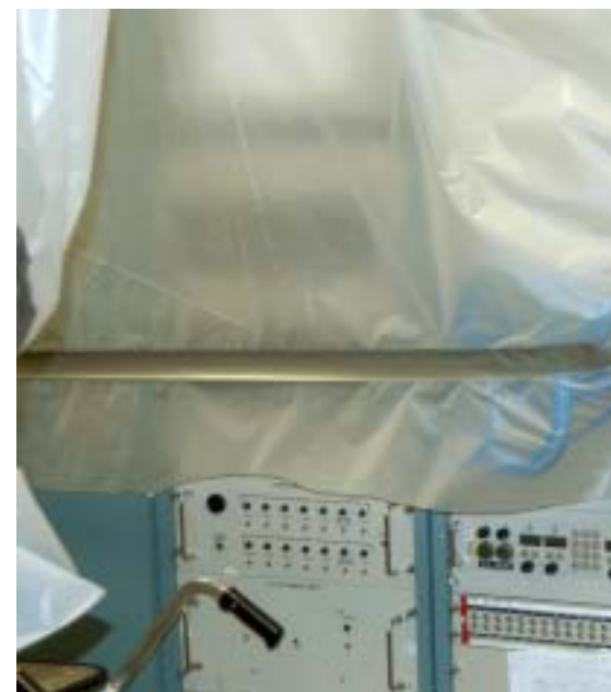
A WORKER COVERS large pieces of equipment in the Complex 39 Area in preparation for the arrival of Hurricane Jeanne.
