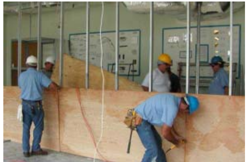
KSC DIRECTOR Jim Kennedy appreciates the hurricane recovery efforts of all Spaceport employees, including these workers rebuilding the Thermal Protection System Facility that lost its roof.
