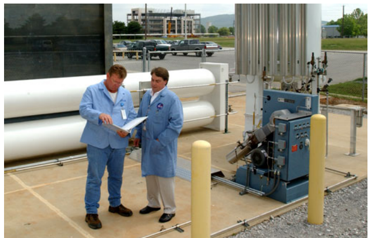
Lead technician Dean Byess, left, and lead engineer Steve Herald go over some technical points at the new LOX/GOX generator system. This is the first system of its kind to be built at Marshall.
