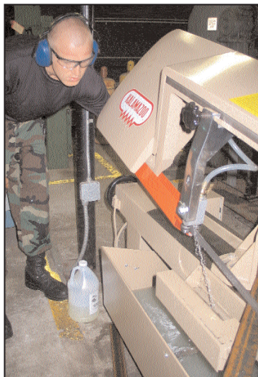
Senior Airman Patrick Rollins, 45th CES structural technician, saws a piece of angle iron he will use to repair storm grates.
