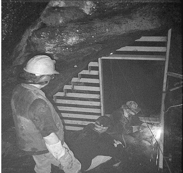
Volunteers from caver organizations have helped install many cave gates in the Ozark Plateau region. Photo by Steve Hensley.
