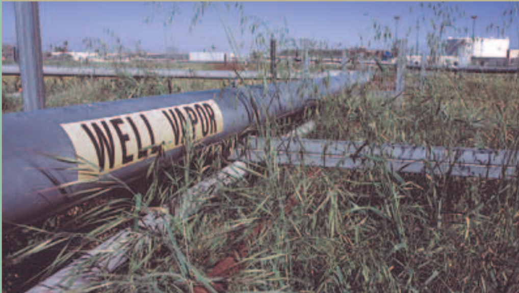
Bill Gendron and Greg de la Paz perform routine maintenance on the Dual Phase Vacuum Extraction system at Los Alamitos Training Center, California.
