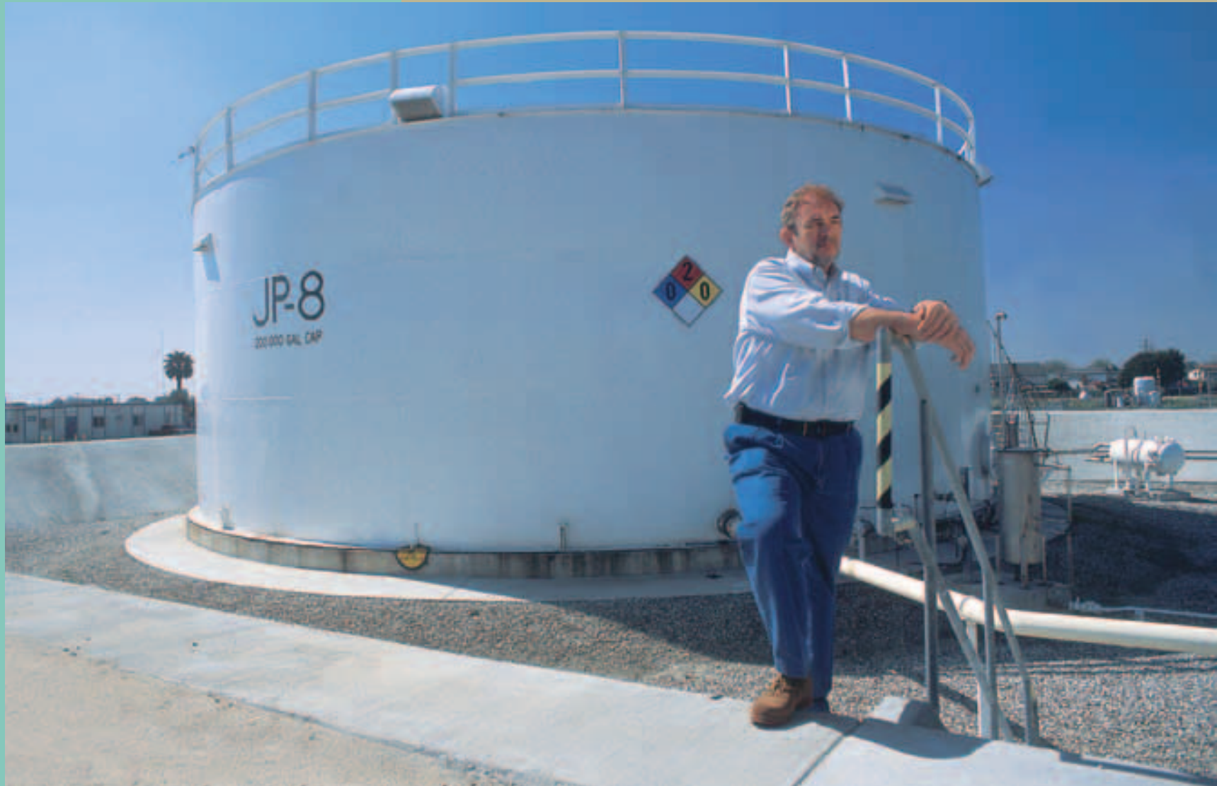
Troy Hardin, environmental manager at Los Alamitos Training Center, California, stands by the National Guard's state-of-the-art, 200,000-gallon above-ground JP-8 fuel storage tank.
