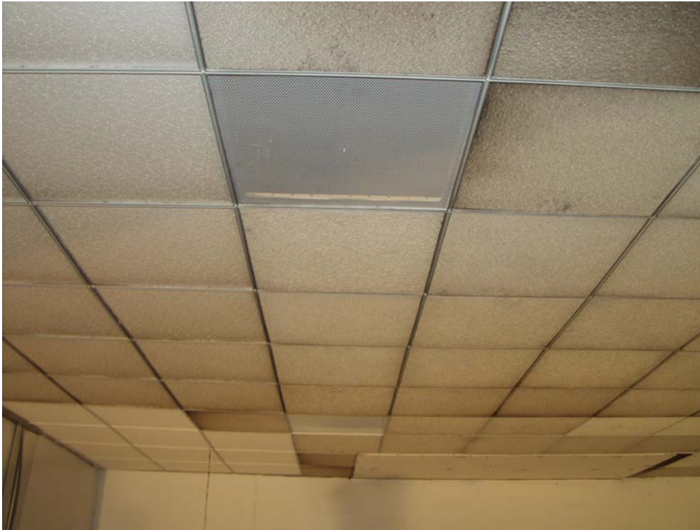
Figure 78. Photograph of the northwest ceiling vent (foreground) and the northeast ceiling vent (rear)
