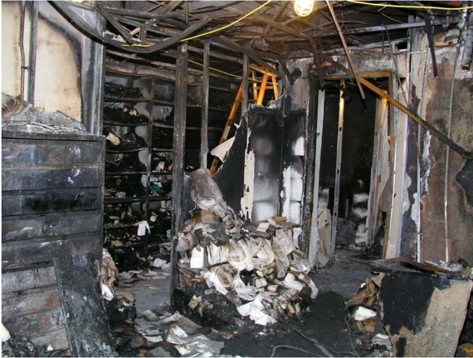
Figure 11. Looking towards the storage room from the open plan office area of Suite 1240
