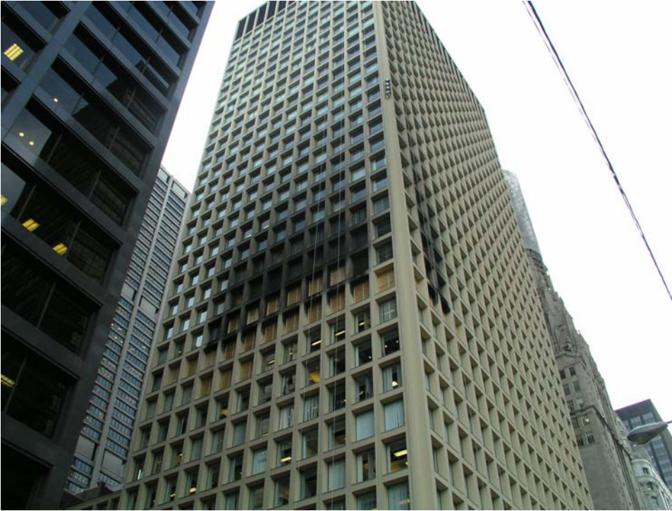
Figure 3. The northeast corner of the Cook County Administration Building, 12 days after the fire
