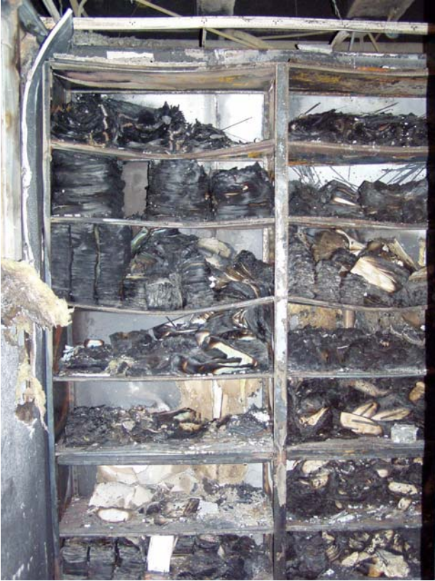
Figure 9. Looking south through the storage room doorway, east end of shelf units
