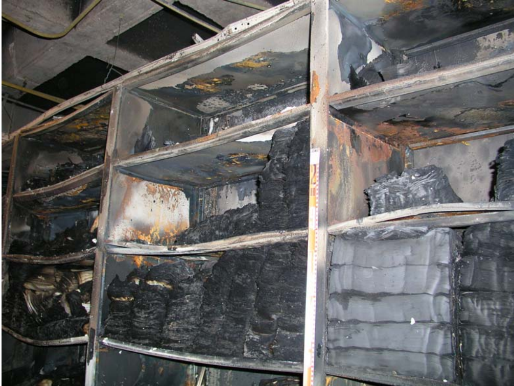
Figure 117. Material on storage room shelves after fire
