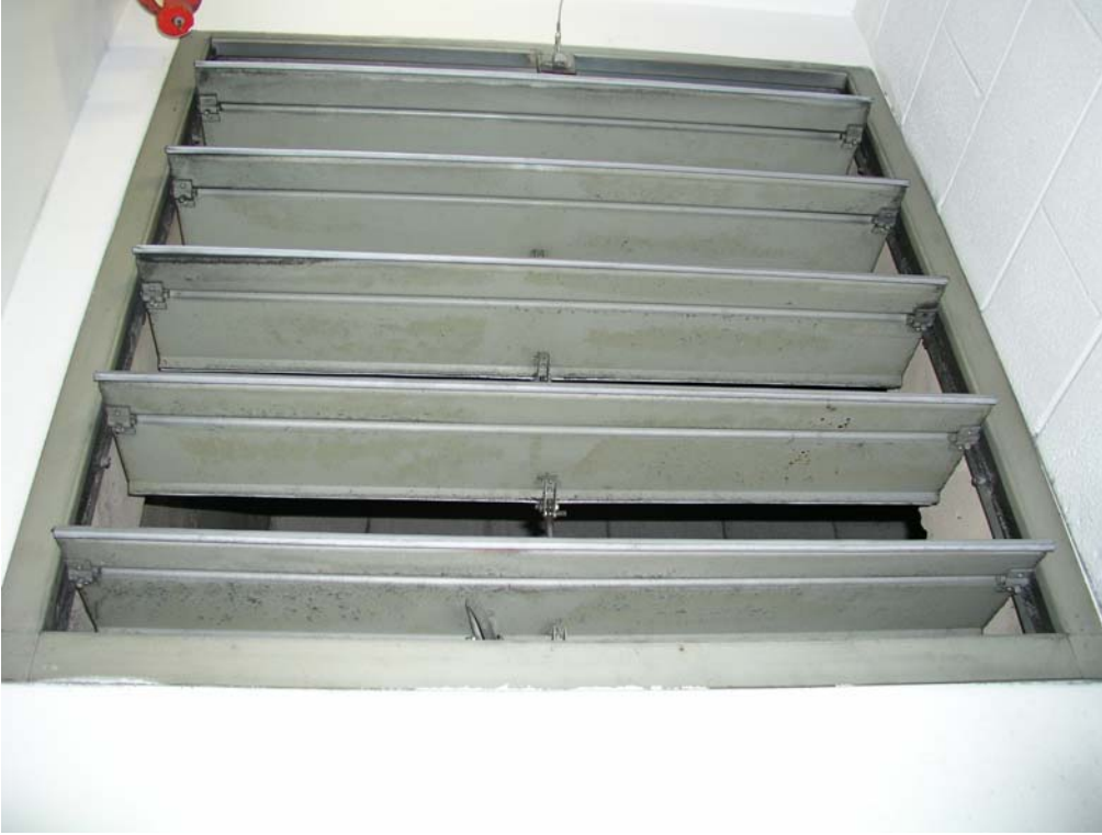
Figure 146. Smoke shaft vent with louvers open
