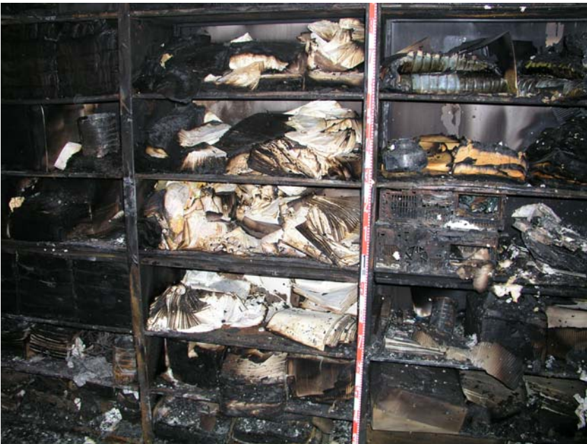
Figure 10. Looking south in storage room, from south corridor (corridor wall removed), west end of shelf units
