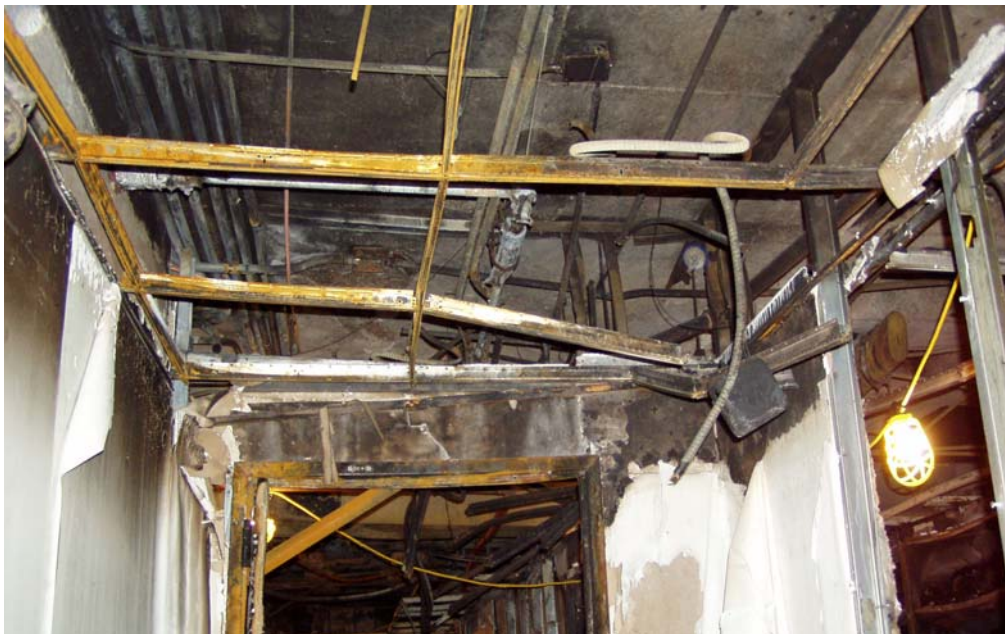
Figure 8. South Corridor looking east toward Suite 1240 doorway. The area of fire origin, the storage room, is on the right
