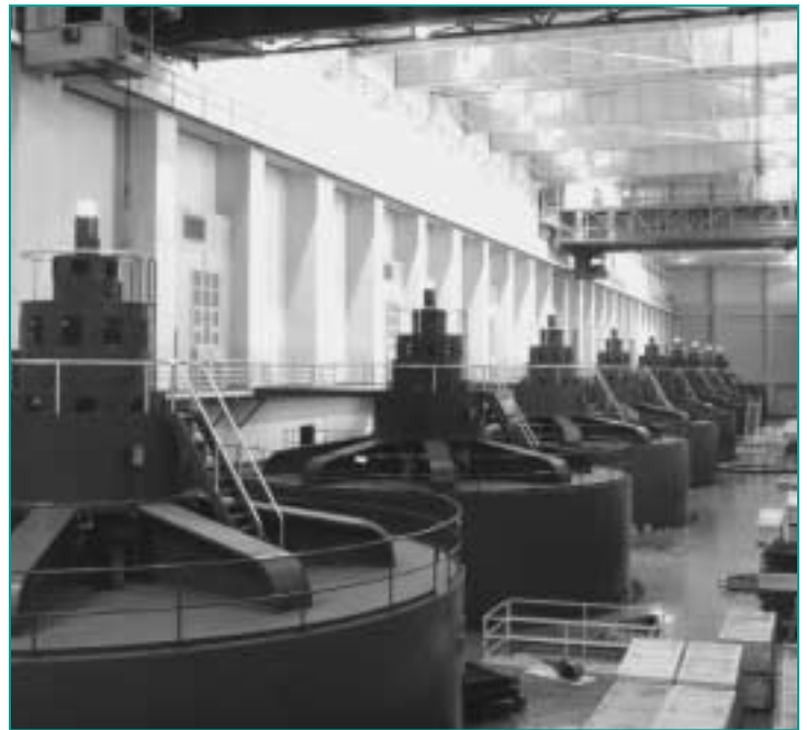
Coordination allows generators to plan routine maintenance at individual plants, such as Bonneville Dam, without disrupting their ability to serve load.
