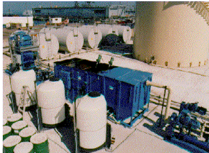
Bilge Oily Wastewater Treatment System (BOWTS).
