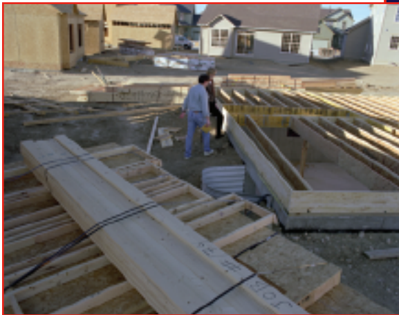
Prefabricated wall panels await assembly at the Meadow View community in Longmont, Colorado. McStain Enterprises is the builder partner.
