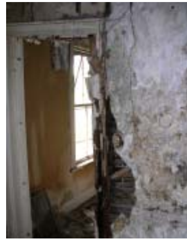
Fig. 6: Deteriorated painted surfaces might pose a health risk during rehab.
