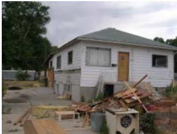
Fig. 4: The demolition of the interior spaces of this home has provided construction materials that can be reused in the rehab project, thereby saving on material costs.
