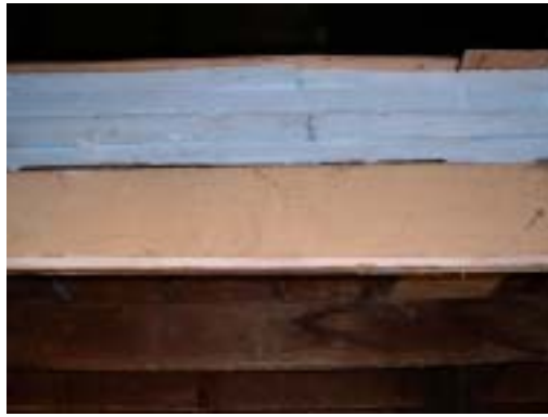
Fig. 27: 4 layers of 2" rigid insulation (Total R=40) installed on the attic floor. Joints between insulation boards should be staggered.
