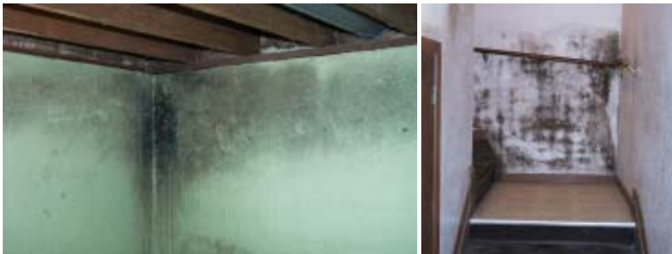
Fig. 7: Mold is a sign that moisture is present.
