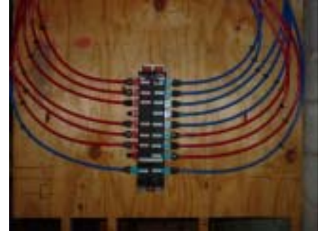
Fig. 36: Manifold water distribution system
