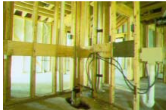
Fig. 10: Installing blocking in walls around tubs and toilets provides the structural support for the installation of grab bars.
