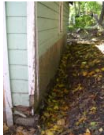
Fig. 12: Improper site grading directed water toward this home.
